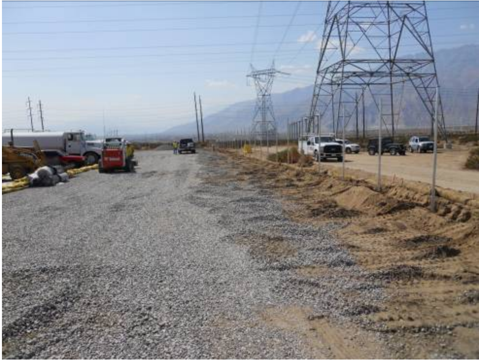
Figure 1: Ongoing construction activities at the Devers Construction Yard include gravel placement and fence installation.
