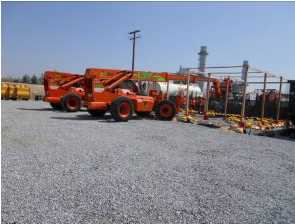
Figure 5: Crews constructing a structure to hold protective bird netting over heavy equipment at the Menifee Construction Yard.
