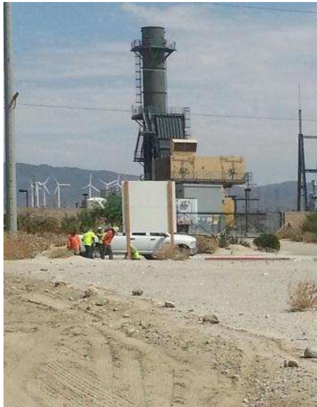
Figure 5. Fugitive dust contact information sign being removed at the Devers 2 Yard as part of the final close-out of the site.
