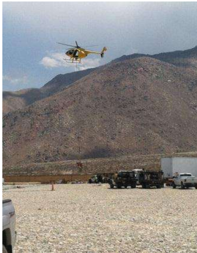
Figure 2. Wire crew members being long-lined from HLZ H1X to Tower 1040 during wire stringing activities.
