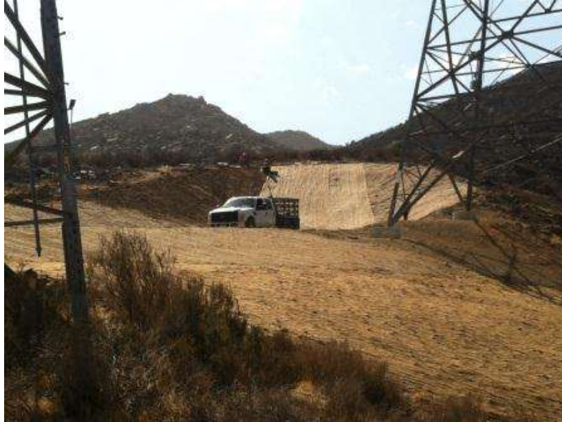
Figure 1. BMP repair at Tower 1081 due to fire damage.
