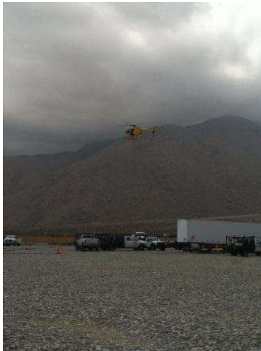
Figure 2. Helicopter work at HLZ H1X for wire stringing activities occurring between Towers 1031 through 1051.
