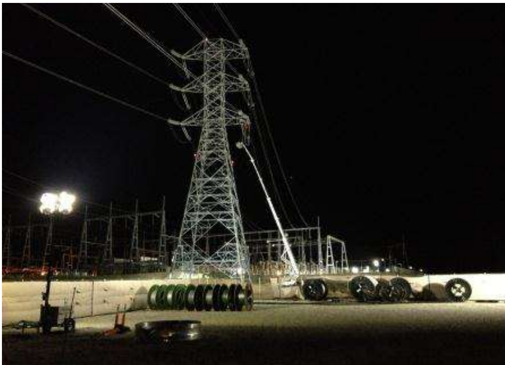
Figure 2. Night stringing work at Tower 1001 and the Devers Substation (Photo courtesy of SCE).
