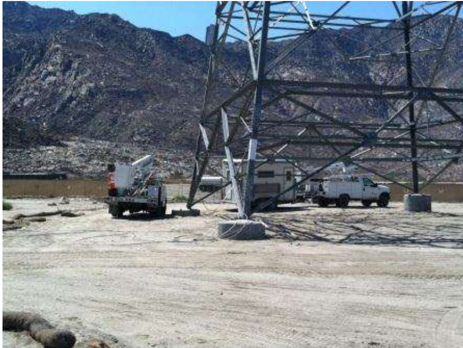
Figure 2. Telecomm splicing at Tower 1051.
