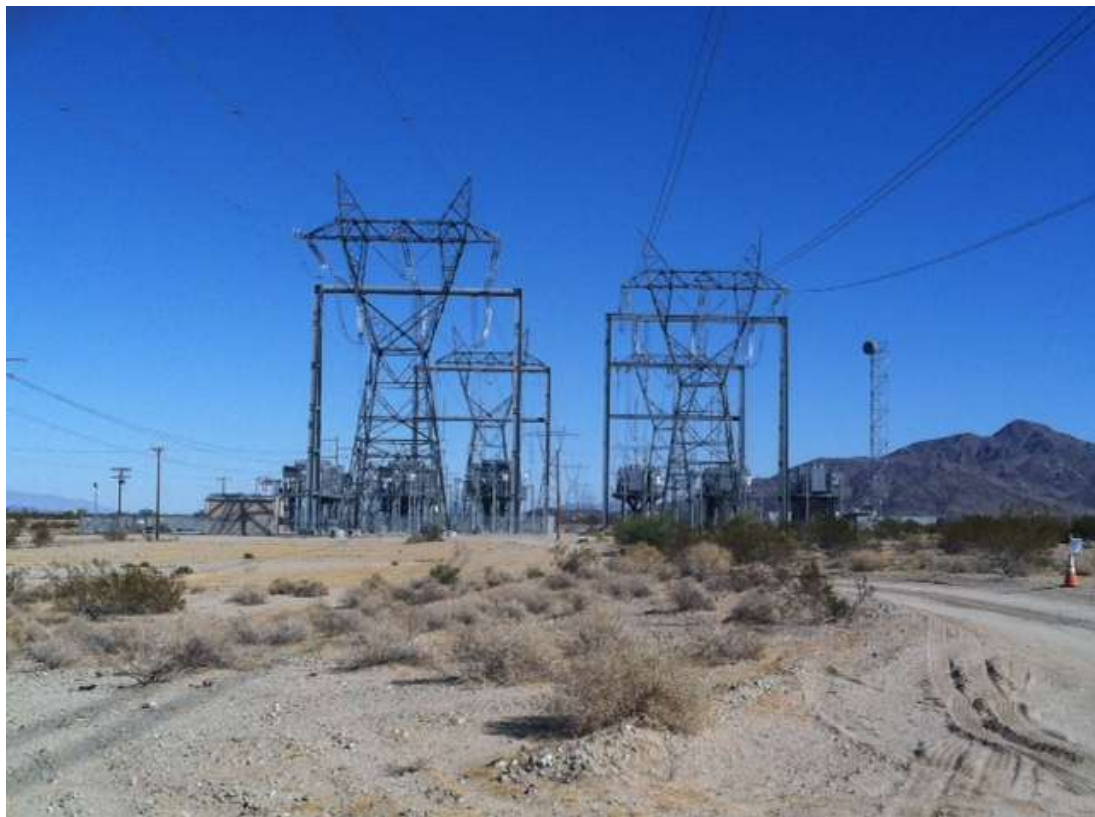
Figure 4. Commissioned Series Capacitor. Please note the construction screening has been removed.
