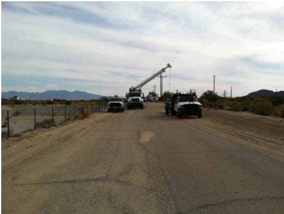
Figure 4: Replacement of old poles with new wooden poles along Aztec Road for the Red Bluff distribution line.
