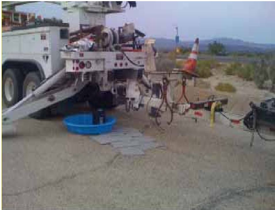
Figure 5: Cleanup of hydraulic leak from the line truck along the Red Bluff distribution line. Note absorbent pads used to remove fluid and pool used to contain additional fluid.
