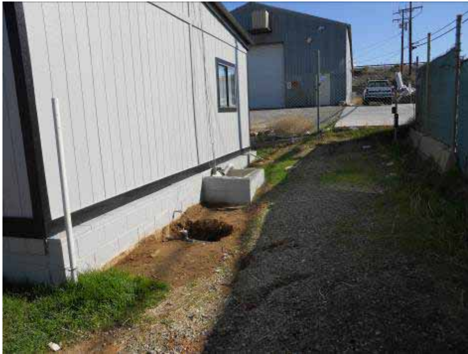
Figure 3: The extent of contaminated soil that was removed as a result of a sewage leak at the Beaumont Construction Yard.
