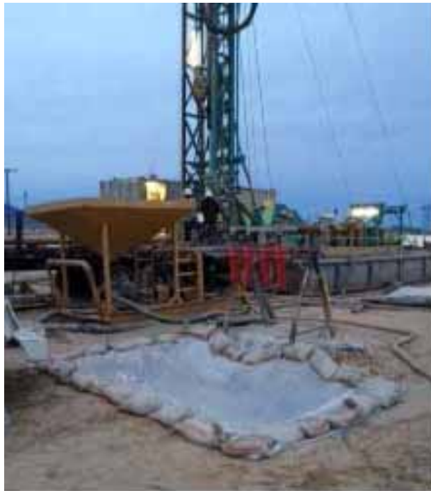
Figure 7: De-sander pit covered at CRS upon the recommendation of the CPUC EM.
