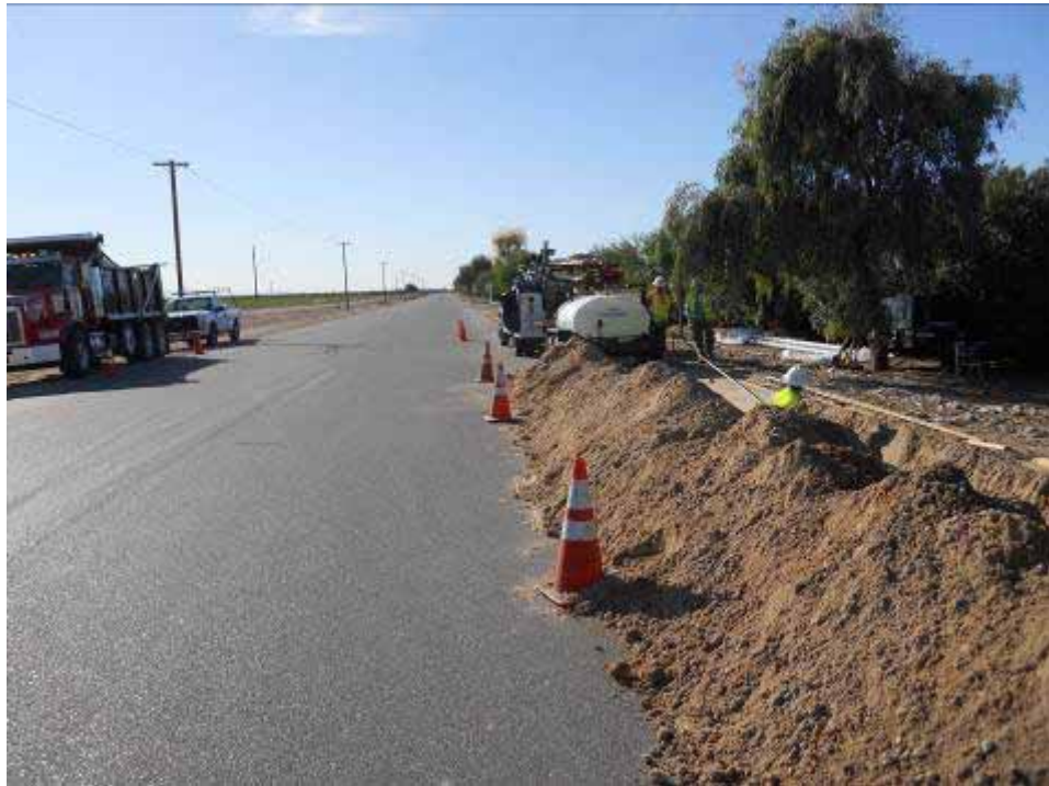
Figure 4: View south along underground portion of the CRS distribution alignment adjacent to Buck Substation.
