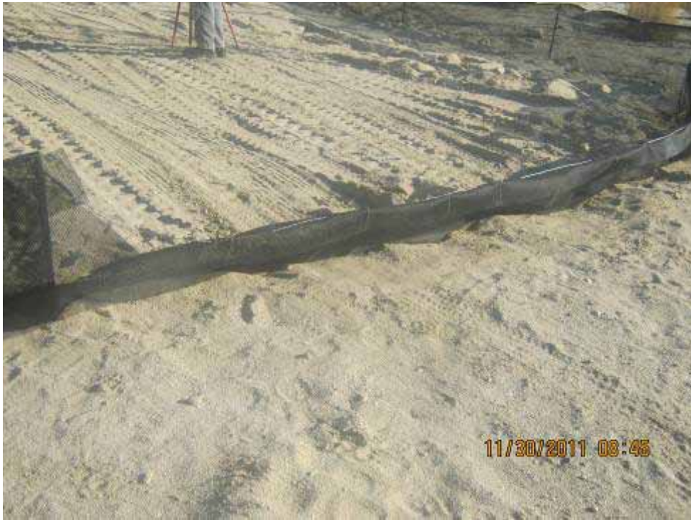
Figure 3: Damaged exclusionary fencing along northern boundary at Tower #2133.
