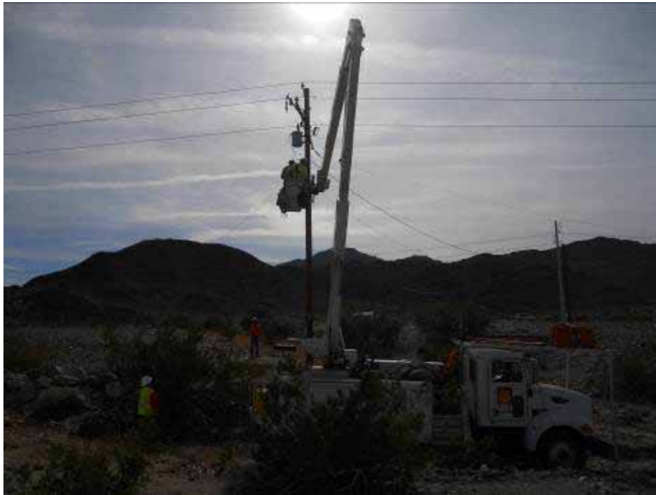
Figure 7: Line crew clipping in new wire along the Red Bluff distribution line (on BLM lands).
