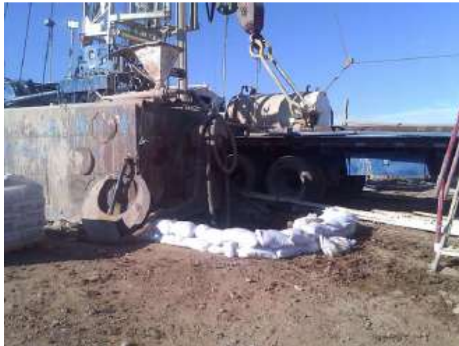
Figure 8: Containment of water leak using sandbags at the Red Bluff Substation drill site.
