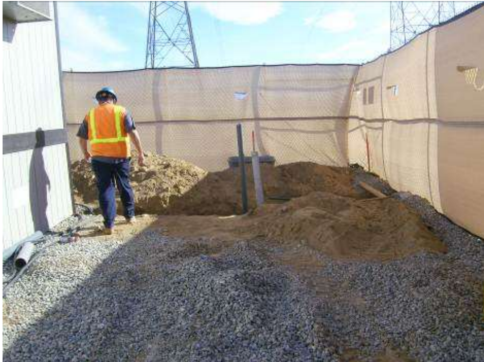
Figure 1: Underground trenching for temporary power at the Devers #1 Construction Yard had reached the yard boundaries by December 20.
