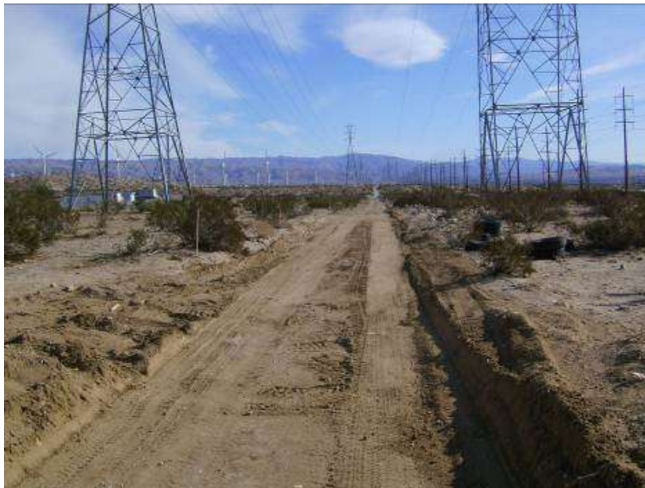
Figure 2: Location along access road at Devers #1 Construction Yard that had been cleaned after underground trenching activities were completed.
