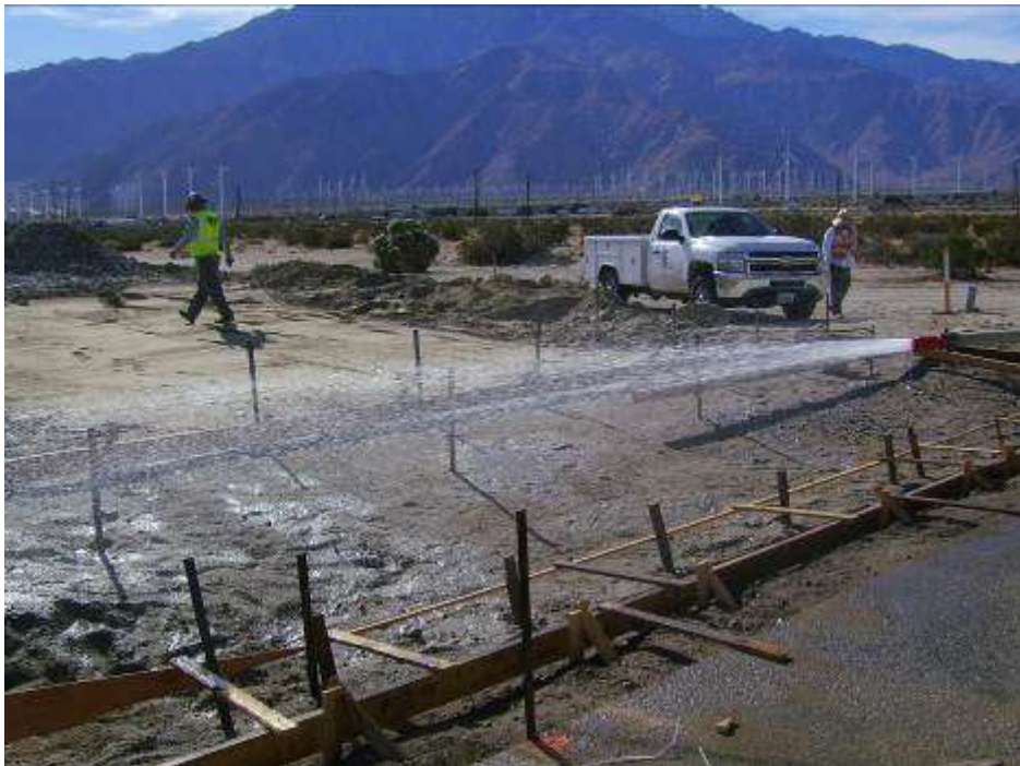
Figure 2: Concrete work being performed at the driveway for the Devers #2 Construction Yard.
