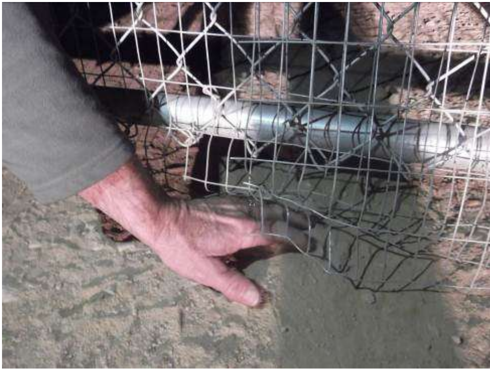
Figure 5. Desert tortoise fencing associated with entrance gate to Red Bluff Substation in need of repairs.
