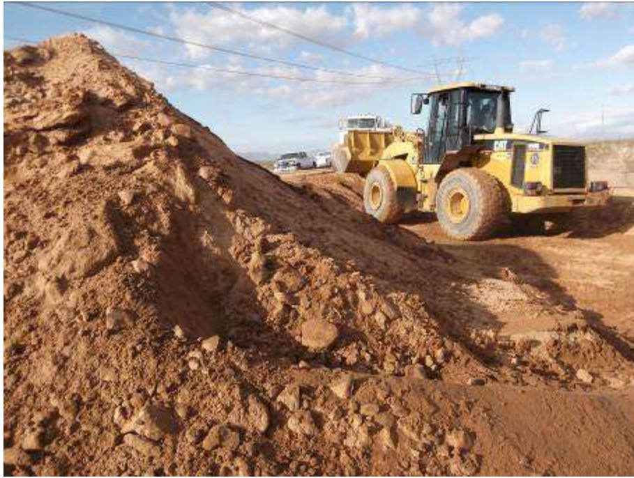
Figure 7. Recontouring activities at the turnout areas associated with the CRS access road.
