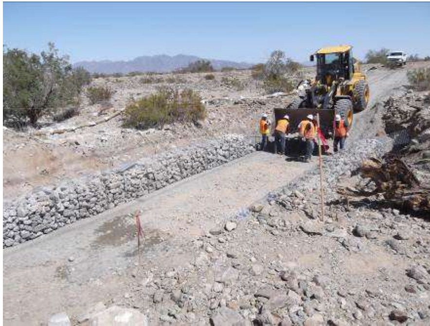
Figure 3. Filling rock gabions at the wet crossing along spur road to Towers RB1-5E and RB2-5E.
