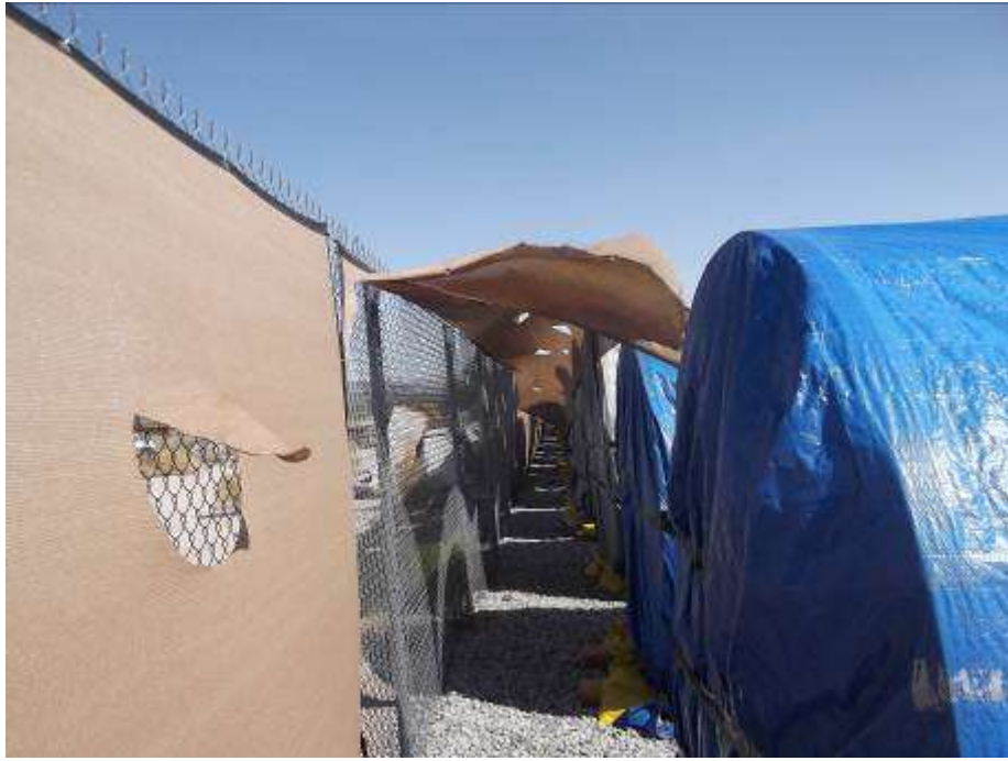
Figure 9. Damaged privacy screening along west fence of Desert Center 1 Construction Yard.
