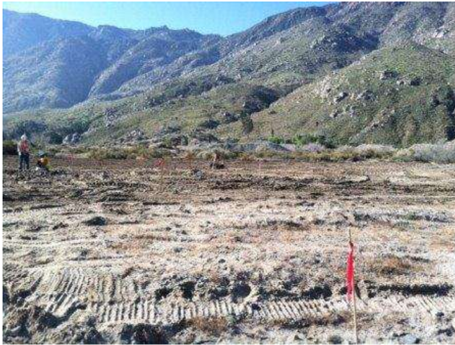
Figure 7. Vegetation clearing, BMP installation, and some grading completed at Tower 1056 prior to site validation by CPUC EM.
