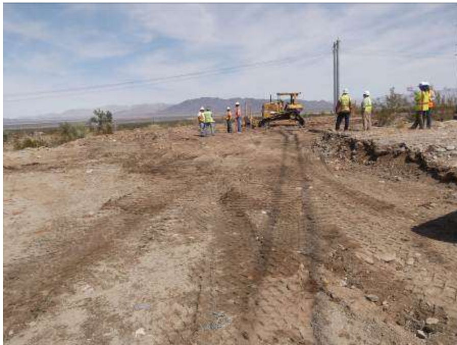
Figure 2. Grading activities nearly completed at Tower 2526. This location is specified for salvage in the Desert Pavement Plan, which was not considered prior to the completed grading work.
