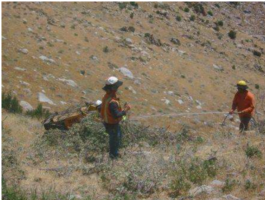
Figure 6. Vegetation clearing activities at Tower 1039. In the photo the Fire Patrol is seen watering down vegetation prior to it being loaded into the vegetation chipper.
