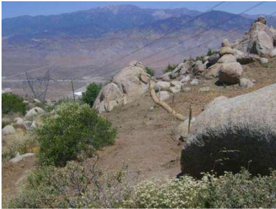
Figure 7. Repairs to RCA at Tower 1047. In the photo the BMPs are placed just outside the RCA and chipped vegetation has been removed.
