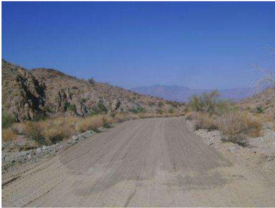
Figure 9. Road base installed on access road just south of Tower 2310 in an area not yet reviewed and released by the CPUC.
