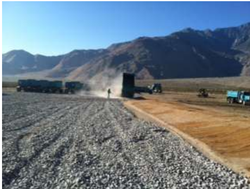
Figure 2. Installation of gravel at the H1X Landing Zone. The gravel is being used as a BMP to prevent fugitive dust at the site.
