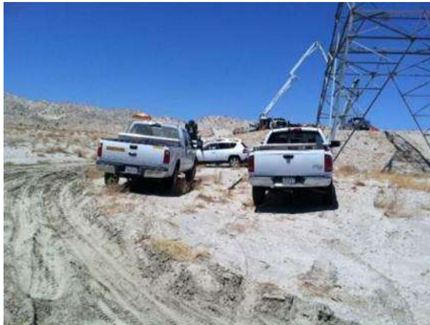
Figure 5. Vehicles parked outside of the approved access road or disturbance limits at Tower 2120.
