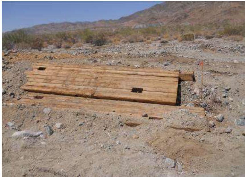
Figure 3. Inadequate foundation hole covering at Tower 2323. Note open holes in wood planks allowing small wildlife to enter and become trapped.
