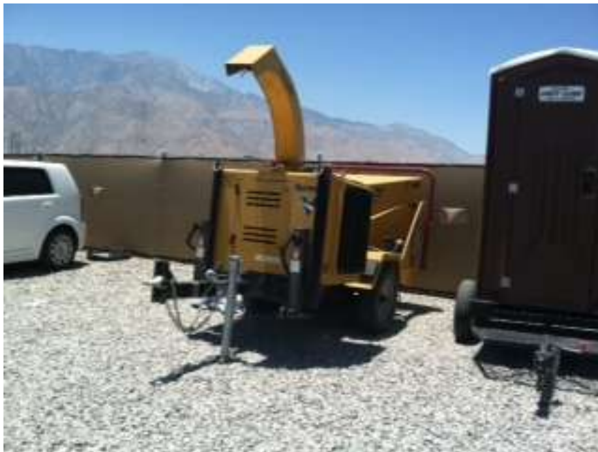
Figure 10. Vegetation chipper staged at the Devers 2 Construction Yard without proper secondary containment.
