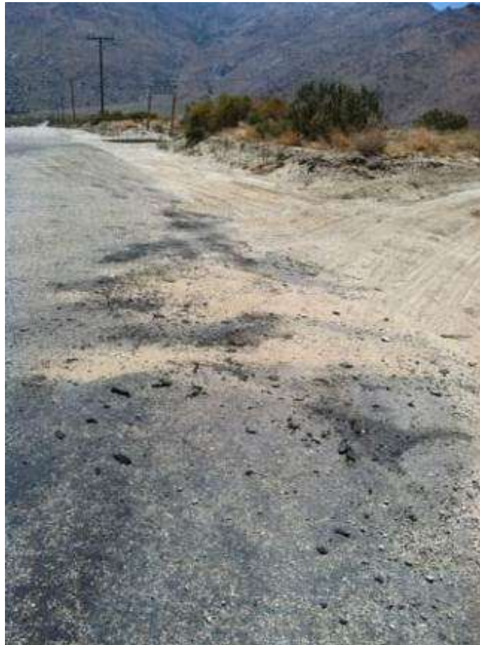
Figure 4. Damage to Snow Creek Road from equipment mobilization near Tower 1029 (photo courtesy of FRED).
