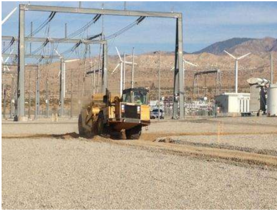
Figure 7. Grading activities conducted within the Devers Substation for a new access road. Photo courtesy of FRED.
