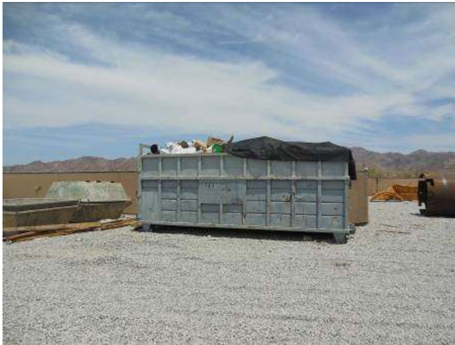
Figure 8. Improper covering of trash bin at Chiriaco Summit Construction Yard.
