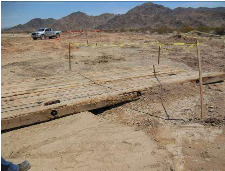
Figure 4. Improper excavation covering at Tower 2437. Note open gap that provides potential for wildlife to enter and fall.
