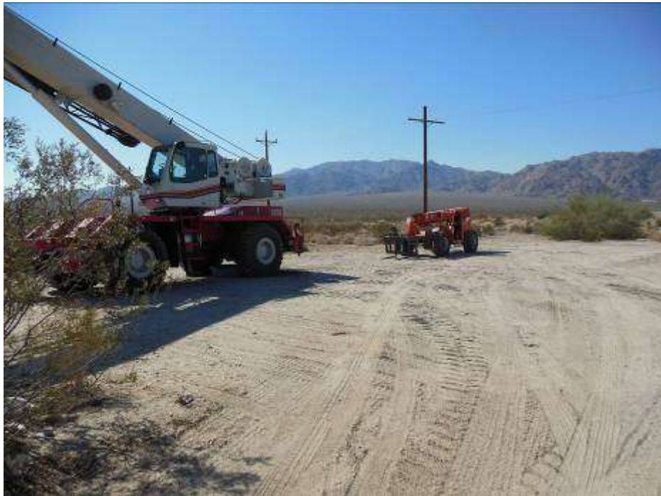
Figure 5. Crane and forklift parked in an unapproved area for staging equipment near Hayfield Road.
