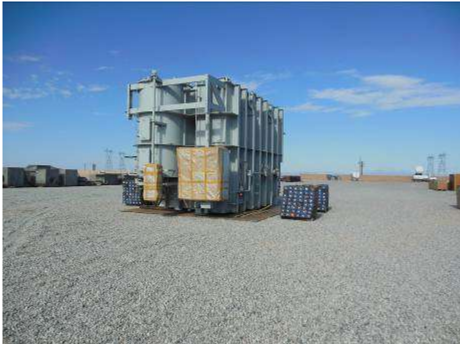
Figure 6. As part of the Package 2 construction phase, the first of four transformers was delivered to the CRS site during the subject period.
