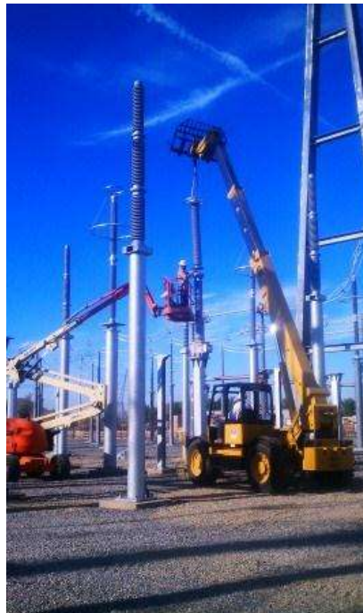
Figure 10. Installation of conductors and insulators at the Valley Substation. Photo courtesy of FRED.
