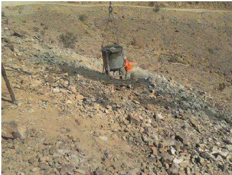
Figure 8. Grout spill at Tower 2310X. Photo courtesy of FRED.
