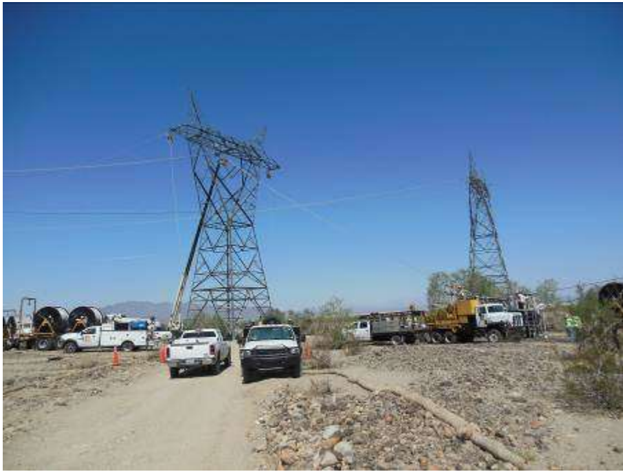
Figure 5. Stringing of Red Bluff loop-in towers with equipment staged at Wire Site RB-11.
