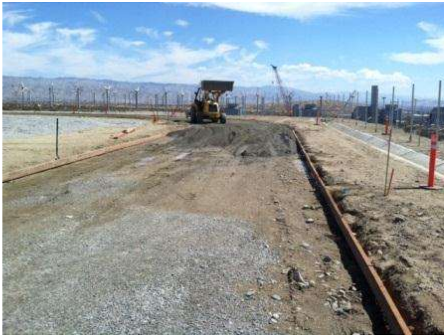
Figure 9. Installation of road base prior to natural pavement at the Devers Substation.
