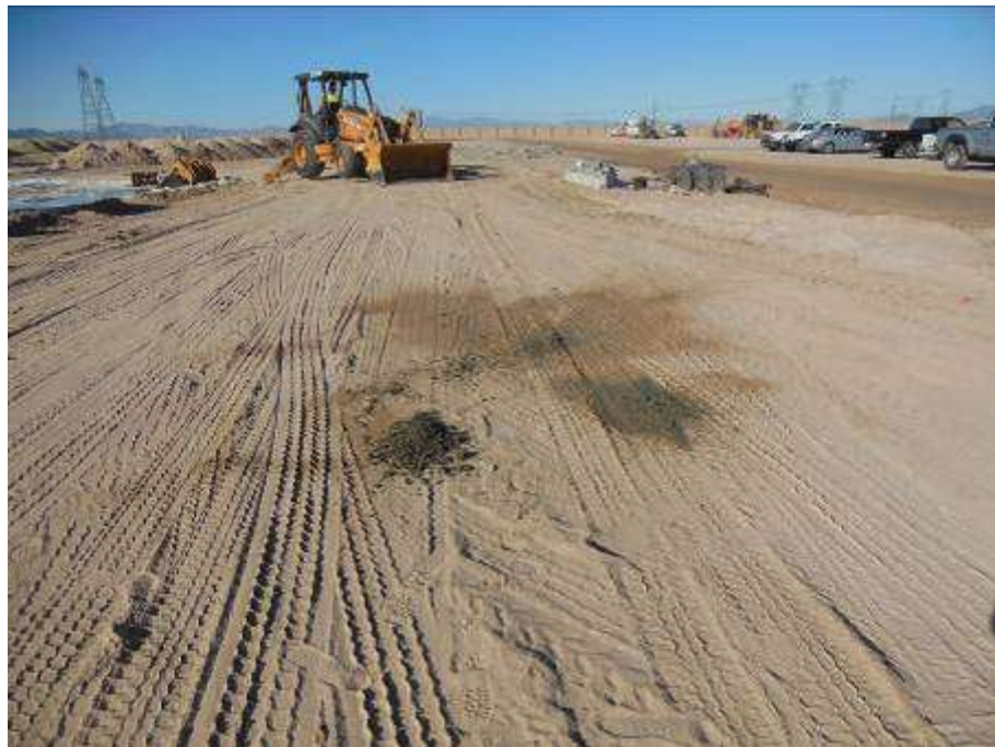
Figure 10. Non-reportable concrete spill at CRS. Remedial efforts were immediately implemented.
