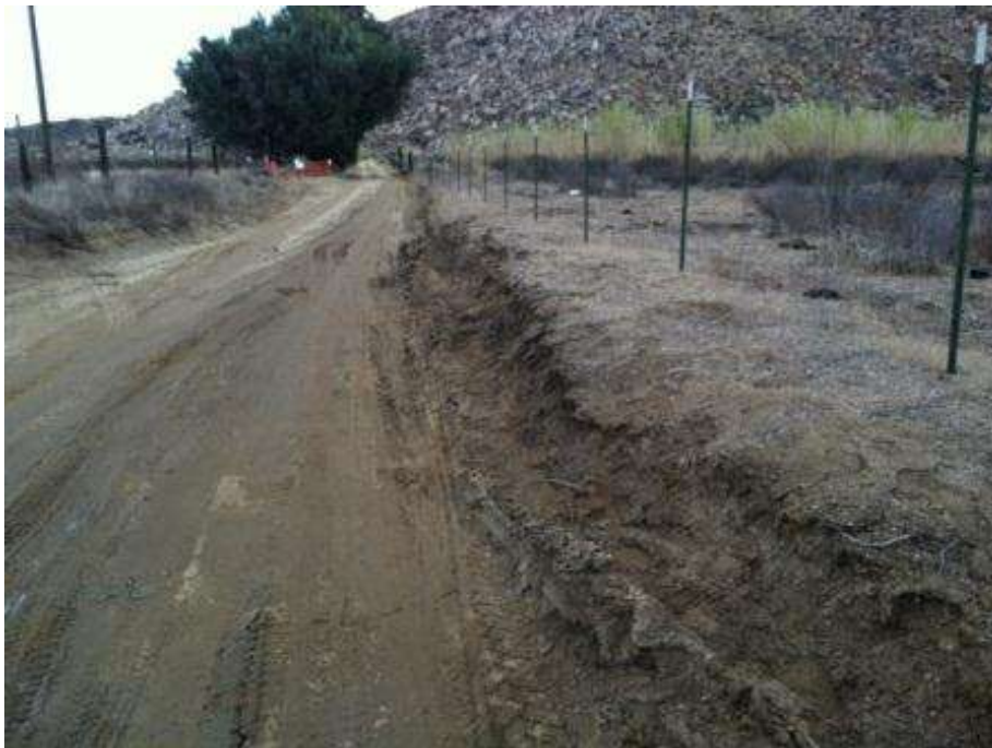
Figure 8. Off-road impacts created by a crane going outside of the approved road limits near Tower 1084.
