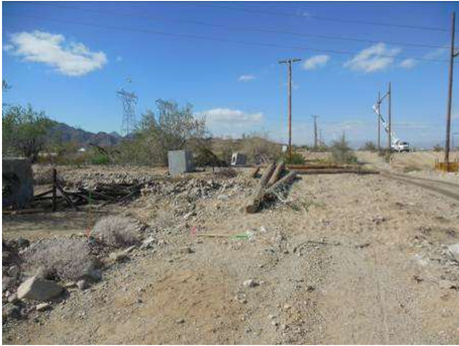
Figure 7. Due to high winds during the evening of November 8, one of the wooden pole structures at Guard Structure RB-06 collapsed. To prevent damage from other nearby guard structures to the existing distribution line that the structures were protecting, the PAR wire pulling crew used multiple fork lifts to knock the structures to the ground.
