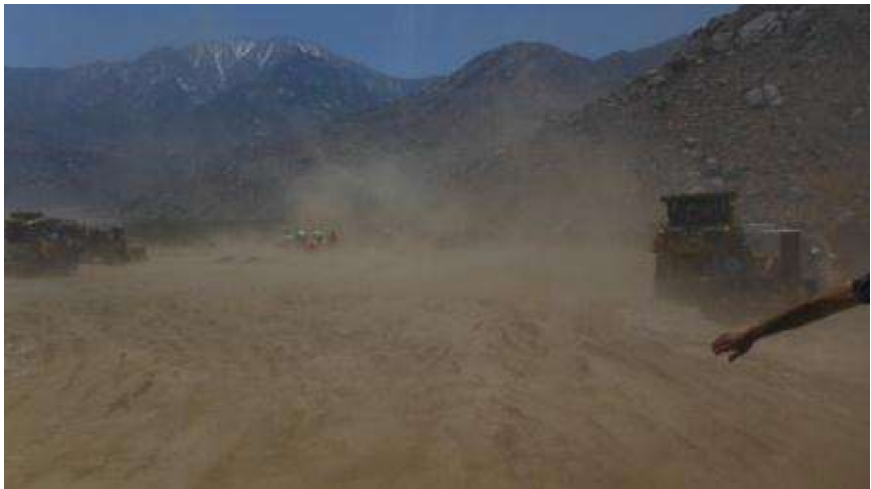
Figure 6. Fugitive dust emission at Wire Site 10 (near Tower 1031). Photo courtesy of FRED
