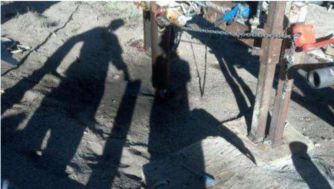
Figure 7. Hydraulic spill at Tower 1042.
