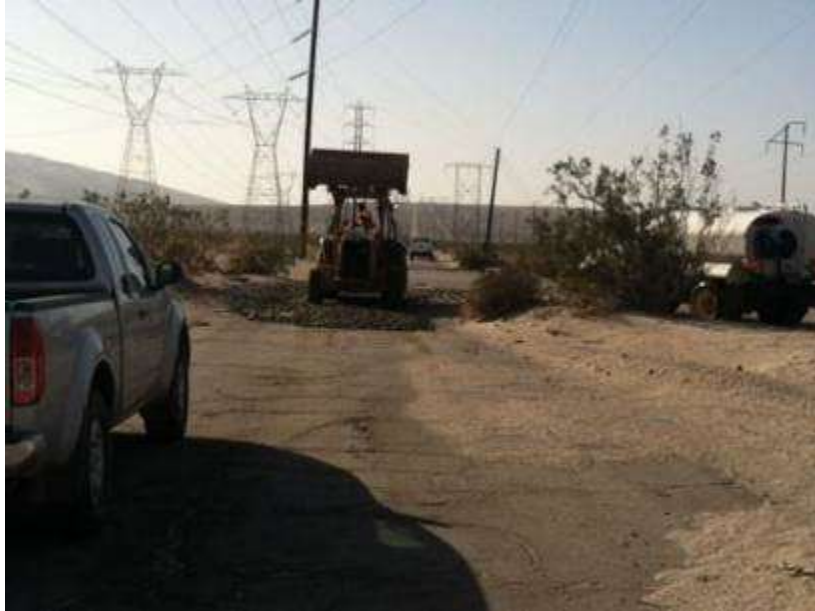
Figure 1. Maintenance of construction entrance at the ROW and Palm Avenue near Tower 2101.
