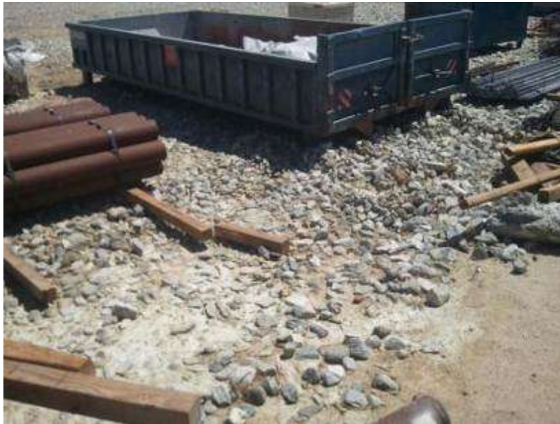
Figure 3. Concrete spill at HLZ H1X.
