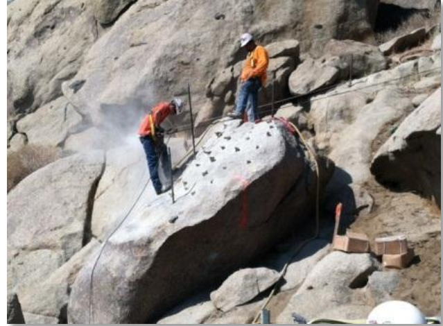
Figure 1. This boulder at Tower 1034 is being prepared for Dexpan to break up rock.
