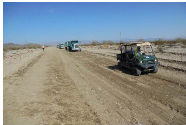
Figure 15. A procession of haul trucks escorted to maintain speed limits along the access road to and from Red Bluff Substation.
