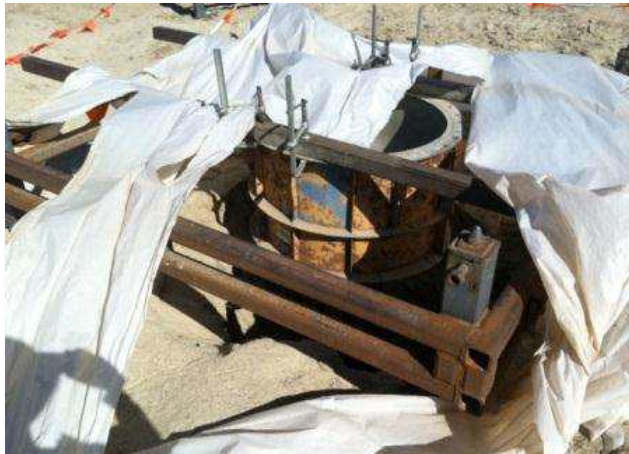
Figure 10. Inadequate covering of open steep-walled excavation at Tower 2126.
