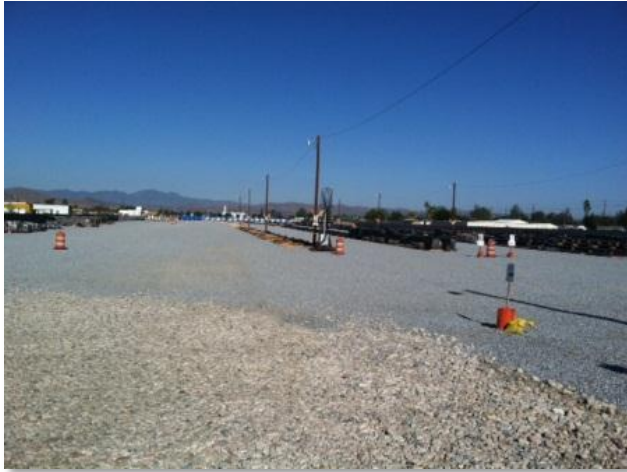
Figure 6. Tower components and equipment storage at the Menifee Yard.
