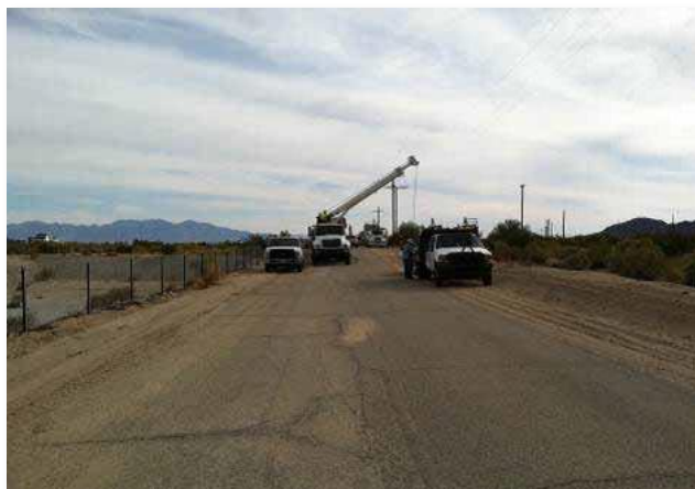
Figure 22. Replacement of old poles with new wooden poles along Aztec Road for the Red Bluff distribution line.
