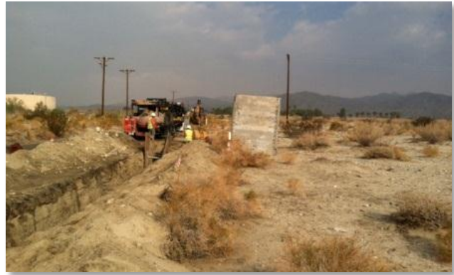
Figure 23. Vault shield placed outside the disturbance area limits at the Mirage Substation Loop-ins project site.
