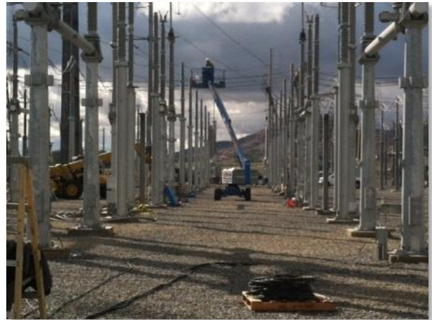
Figure 17. Assembly of circuit breakers and disconnect switches at the Valley Substation.
