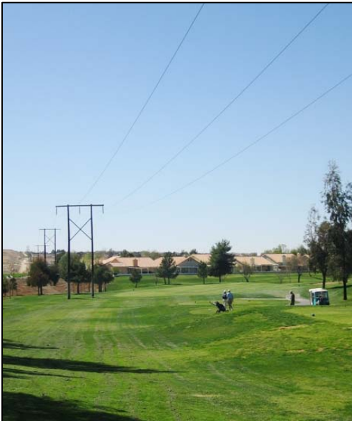
Existing 115 kV Subtransmission Line through the Sun Lakes Community
