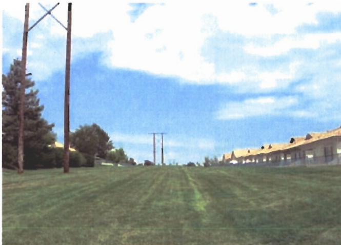
Figure 3A. Looking East from Highland Springs Road Existing 115 kV Subtransmission Line
