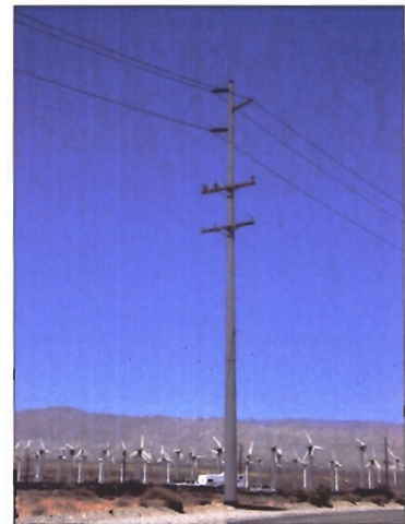
5. Typical new single-circuit pole with distribution underbuild and communication cable
