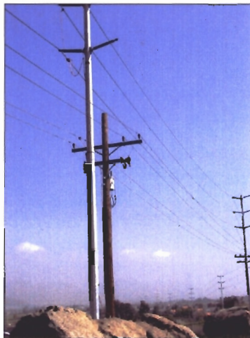
4. Transfer 12 kV or 33 kV wires, install new 115 kV circuit wires, and remove old pole
