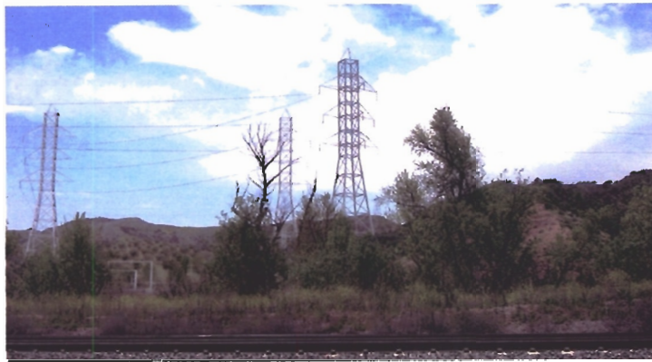
Simulated view of El Casco Substation Site from San Timoteo Canyon Road (Key View 3)
