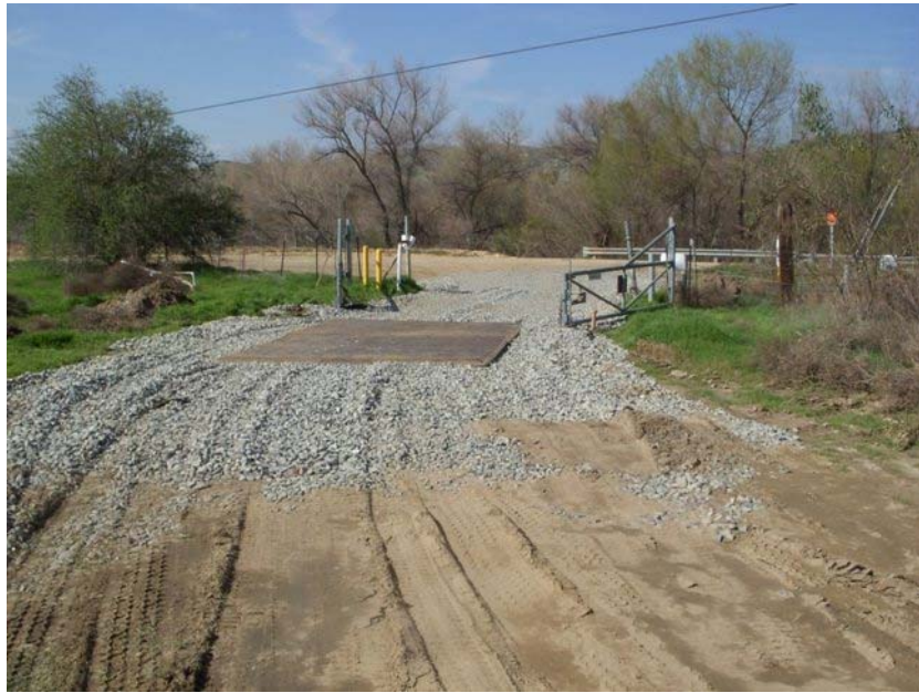
Figure 7: A gravel bed and a shaker plate were installed at the entrance of the access road to San Timoteo Canyon Road to reduce dirt from project vehicles entering the public roadway. The photograph faces northwestward.
