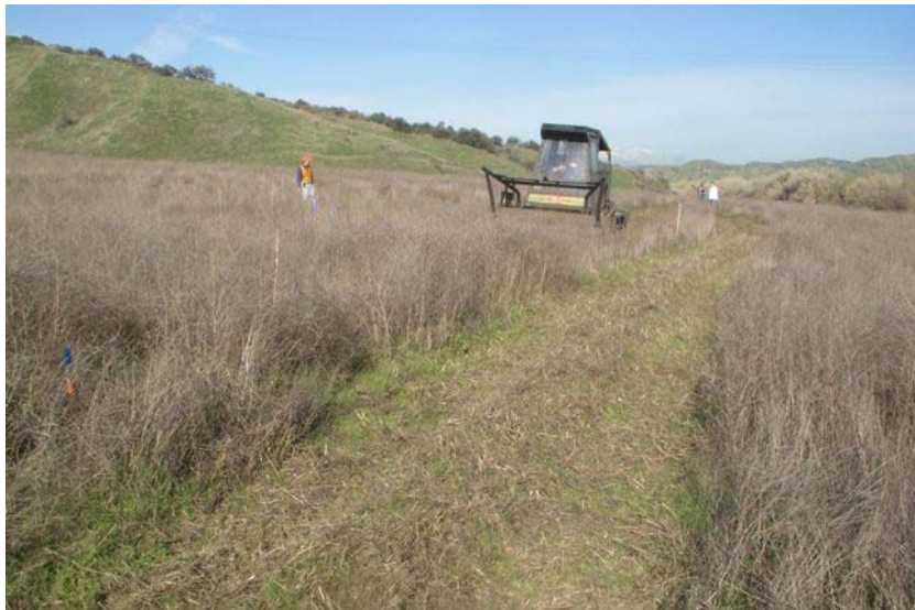
Figure 4: The lower, level portion of the substation site which was vegetated with non-native grass and other ruderal herbaceous vegetation was mowed by Wendy's Tree Service and its subcontractor, BZB. One or more cultural resource consultants and one or more biologists accompanied the two mowing machines at all times during the mowing operation. The photograph faces westward.
