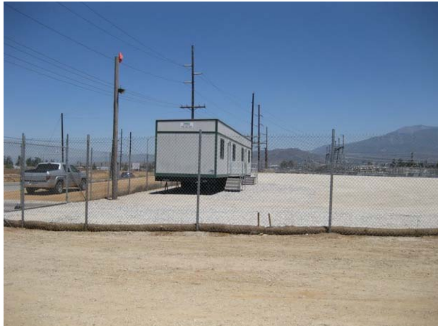
Figure 4: The Maraschino Substation Laydown Yard has been completed. The yard office trailer is on site, but has not been electrically connected and is not yet functional. The south border fence (in foreground) was moved northward thirty-five feet to ensure that the Yard is wholly located on one property. The straw wattling at the base of the south border fence was placed to prevent siltation onto adjacent property. The entrance gate is to the left in the foreground and has an asphalt driveway connecting from Veile Street. The photograph faces northward.
