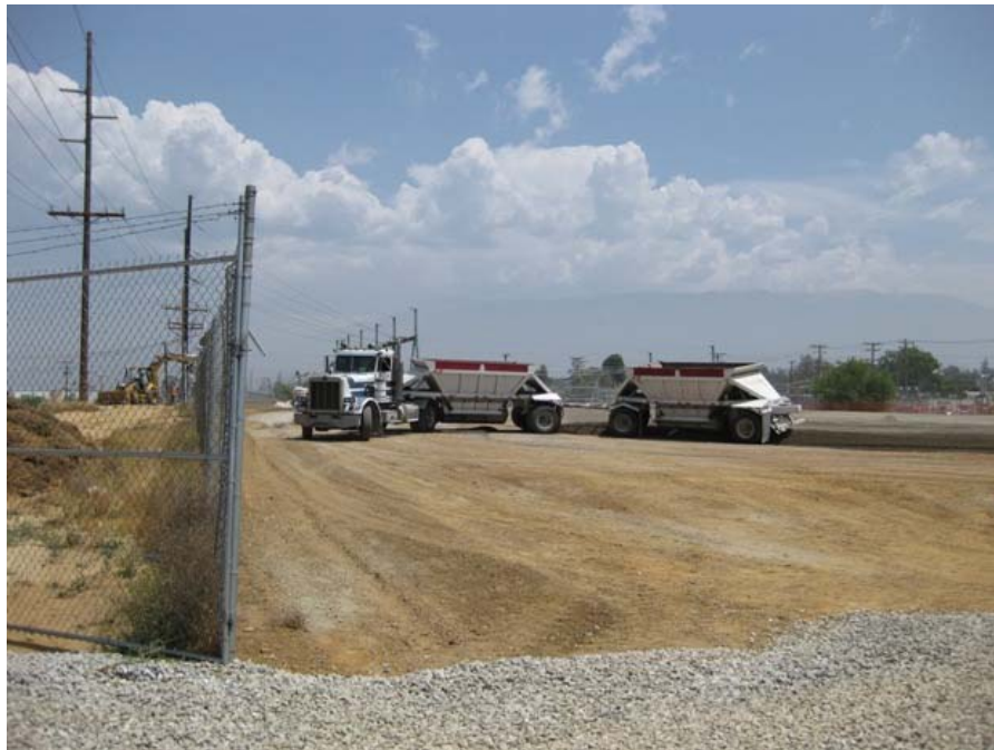
Figure 3: The Maraschino Laydown Yard was prepared by light scraping and removal of vegetation, and hauling in and spreading of gravel base. The photograph was taken during preparation of the yard and faces northward.
