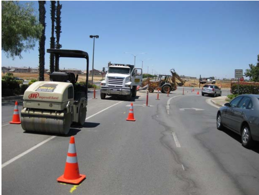
Figure 1: Installation of underground FOC conduit is occurring on First Street in Beaumont and on Sun Lakes Boulevard in Beaumont.
