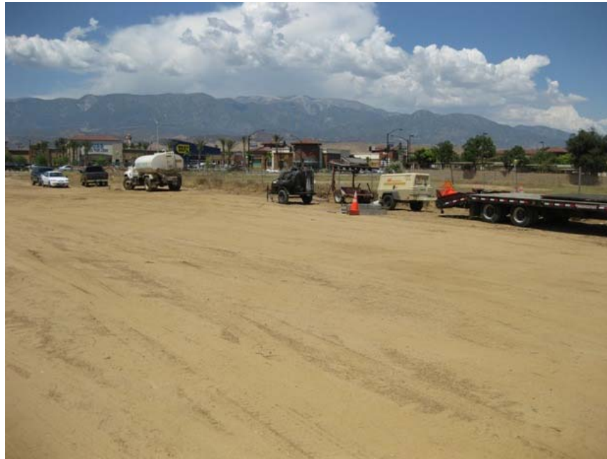
Figure 8: A staging area has been developed for the Sun Lakes fiber optic cable installation in a vacant lot north of First Street and west of Highland Springs Road. The photograph faces southwestward.
