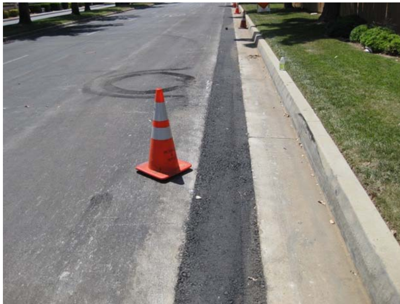
Figure 6: The fiber optic cable is being placed within the roadway at the Sun Lakes development in Banning. The photograph was taken on Sun Lakes Boulevard, and faces westward.
