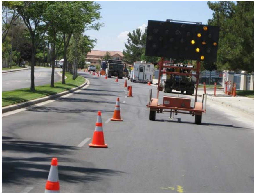
Figure 7: Proper signage, demarcation of the work limits, and traffic control is occurring at the Sun Lakes Boulevard fiber optic cable installation. Steel plates are used to protect the road surface from equipment damage, and to cover open trench. The photograph was taken on Sun Lakes Boulevard and faces westward.
