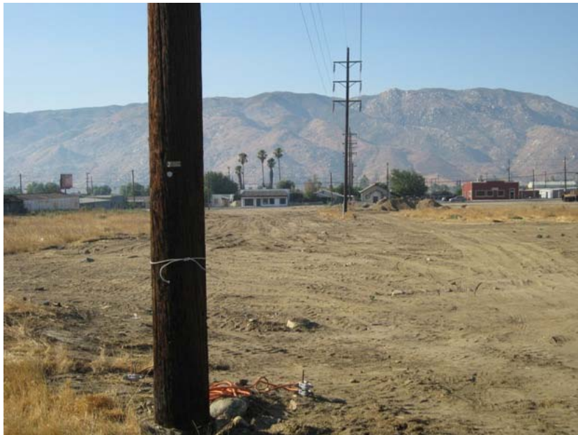
Figure 2: Evidence of work on pole A1320677E of the Devers-Banning-Windpark-Zanja line on the south side of Williams St. in Banning was visible at 0720 hours on August 27, 2009. This evidence included ground disturbance, grounding wires, and temporary wiring at the upper cross bars. The CPUC validation of the pre-construction biological survey had not yet been completed. This pole was incorrectly identified as being on the north side of Williams St. in the NTP #3, MOD #1 request. The photograph faces southward.
