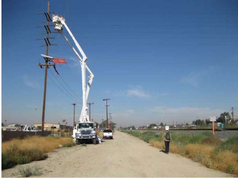
Figure 3: On August 28, 2009, work occurred on pole A1335682E, located at the northwest corner of the Banning substation. A biological monitor from NRC (right side of photograph) was present during this activity). The survey validation had been completed by CPUC on the previous day. The photograph faces westward.
