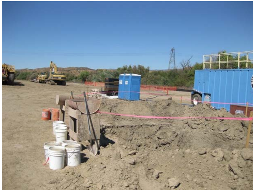
Figure 7: The excavated pit at El Casco Substation site is in the distance behind the orange fence. The blue tank on the right is storing the pumped groundwater. The generator supplying power is the dark structure behind the portable toilets. It has been placed within a spill containment structure.. The photograph faces northwestward.
