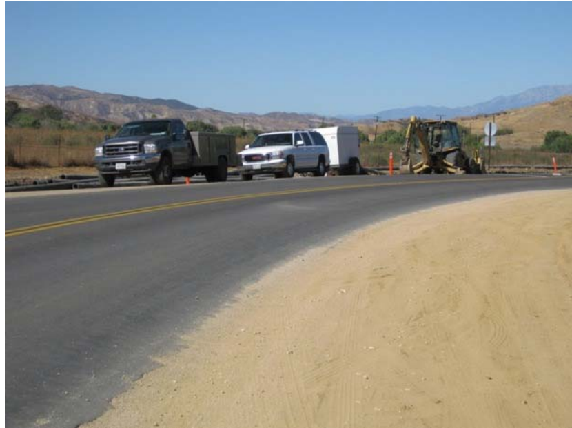
Figure 1: Construction began on the above-ground water pipeline being placed on the south shoulder of San Timoteo Canyon Road between a source well at the Fisherman's Retreat Campground and the entrance gate of the El Casco Substation site. The photograph faces westward.
