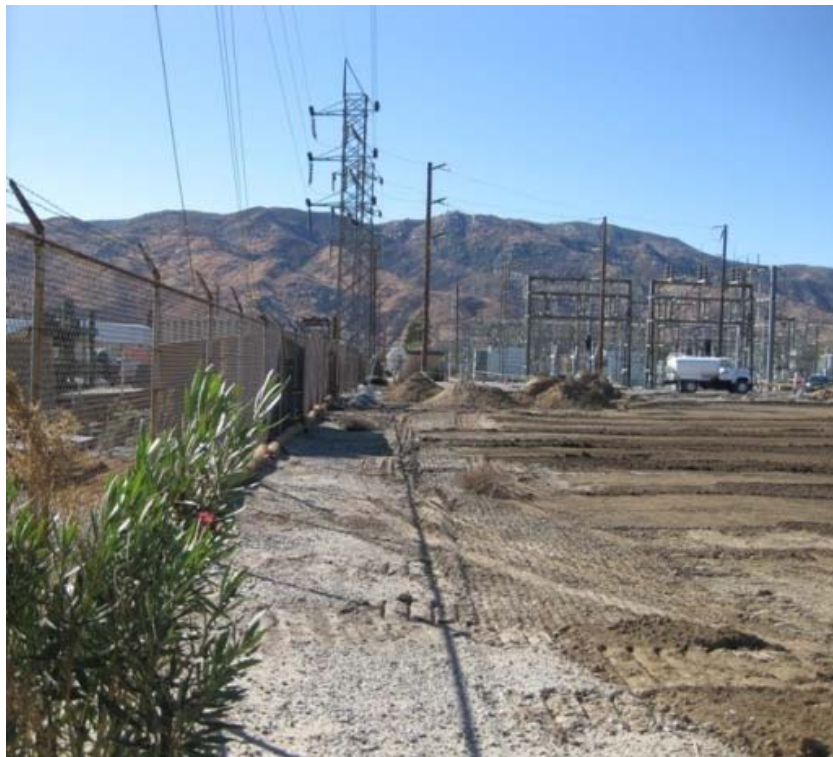
Figure 2: During the subject week, grading began at the Banning Substation in preparation for upgrading. The photograph was taken from the John Street entrance and faces southward.
