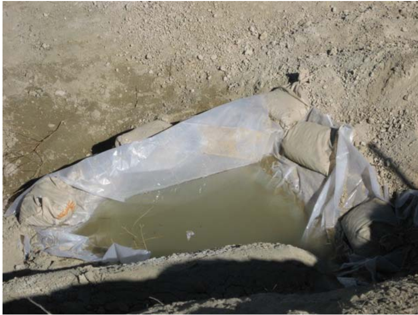
Figure 3: Small concrete wash-out basins were created at each terrace on the hillside at El Casco Substation.
