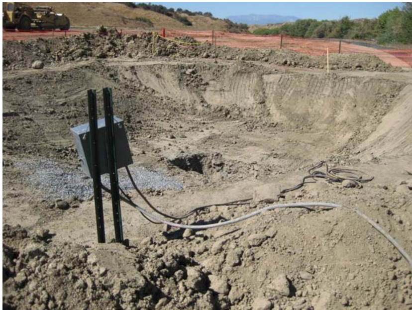
Figure 5: At the El Casco Substation site, a thirty-foot wide pit was dug within twenty-five feet of the San Timoteo Creek bank in order to determine ground water level.
