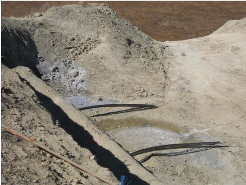
Figure 4: Some concrete spillage occurred at the terraces. The concrete will dry and be buried during the backfill operation.
