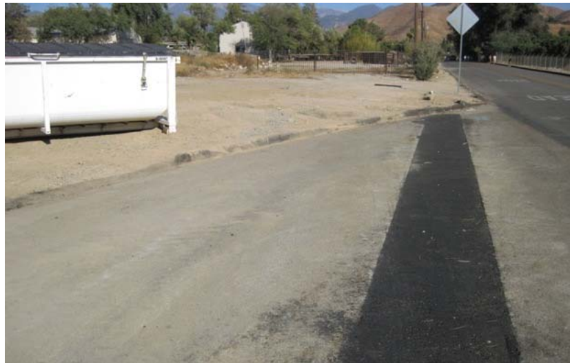
Figure 4: During trenching for installation of underground FOC in front of the Mentone Substation on Monday of the subject week, an unmarked pipe was ruptured just in front of the photograph. The bins on the left contain contaminated soil that was removed. The trench was re filled and paved without placement of the FOC. The unmarked pipe is located on the left side of Colton Street for several hundred feet in the distance. The photograph faces eastward.
