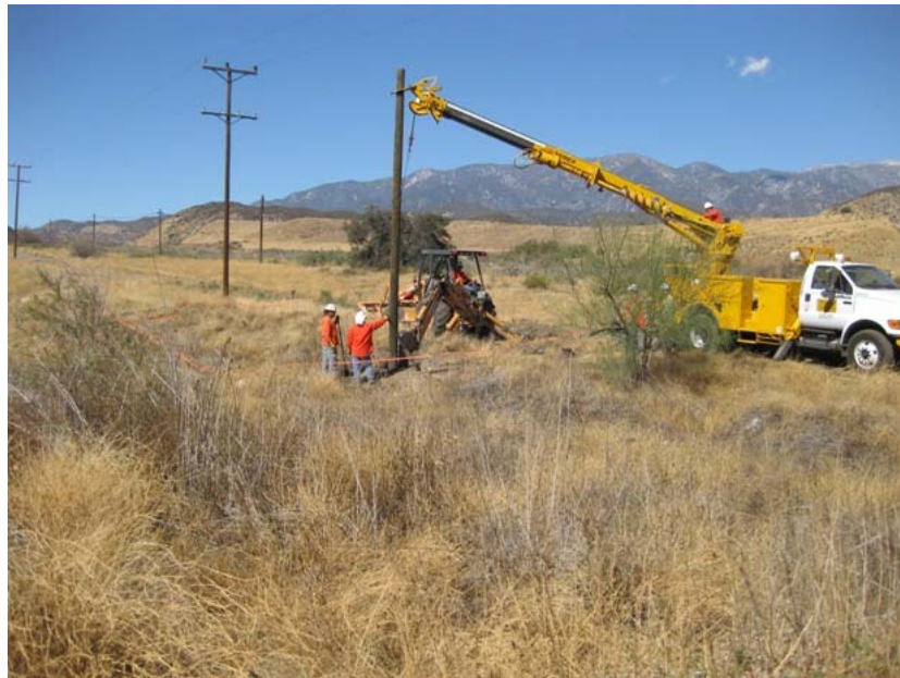
Figure 2: Additional poles were placed in the construction of the temporary Banning shoo-fly FOC route. The photograph was taken east of Bluff Street in the hills north of Banning and faces northward.
