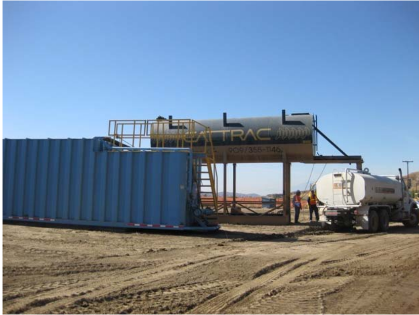
Figure 1: During the subject week, the above-ground water pipeline along San Timoteo Road between a source well at the Fisherman’s Retreat Campground and the entrance gate of the El Casco Substation site was completed, and placed in operation. The water is pumped into the blue settling tank, and then into the raised water tower where Project water trucks are filled. The photograph was taken just inside the Project entrance gate and faces westward.
