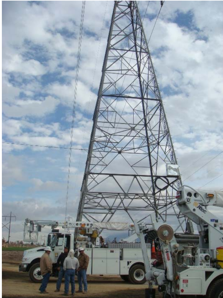
Figure 1: SCE Fiber Optic Cable crews worked on the Calimesa shoo-fly installing cable, and two 3x3 boxes at either end of the shoo-fly. The photograph was taken at the eastern end of the shoo-fly within Oak Valley Golf Course northeast of I-10 Freeway and south of Brookside Avenue, and faces eastward.
