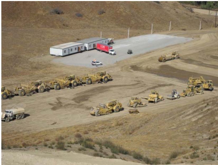
Figure 4: During the subject week, the two SCE project field trailers recently placed on graded sites continued to be readied for occupancy. The equipment yard has been moved out of the over-excavated area to an area further south. The photograph faces northwestward.
