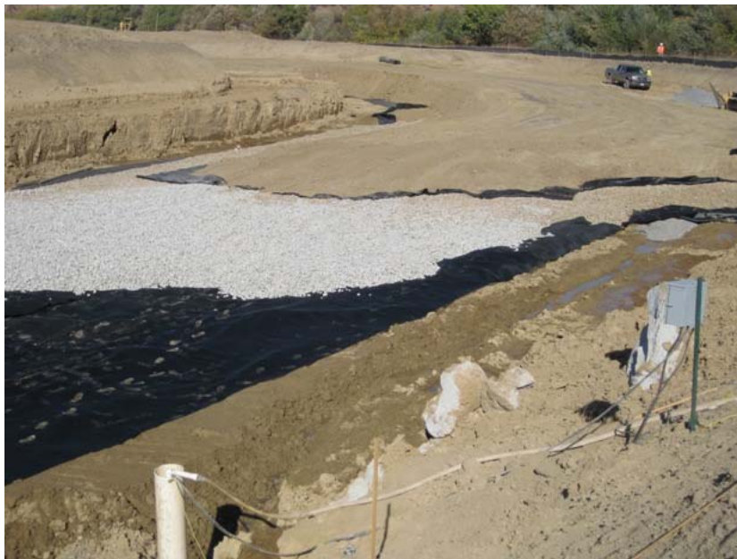
Figure 2: The westernmost over-excavated area of the El Casco Substation site is being lined with water resistant fabric and an underlying gravel blanket. Material from the site will be used as fill and will be compacted to form a firm base for the substation foundation. The photograph faces northward.
