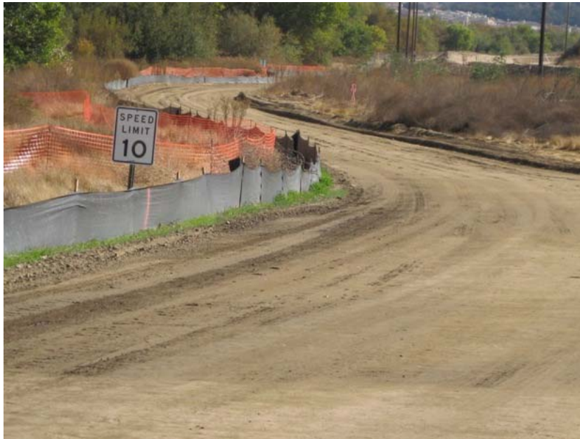
Figure 5: Dust control continued to be maintained throughout the El Casco Substation and access road sites. The ten miles per hour speed limit is being enforced. The photograph faces eastward along the original access road.
