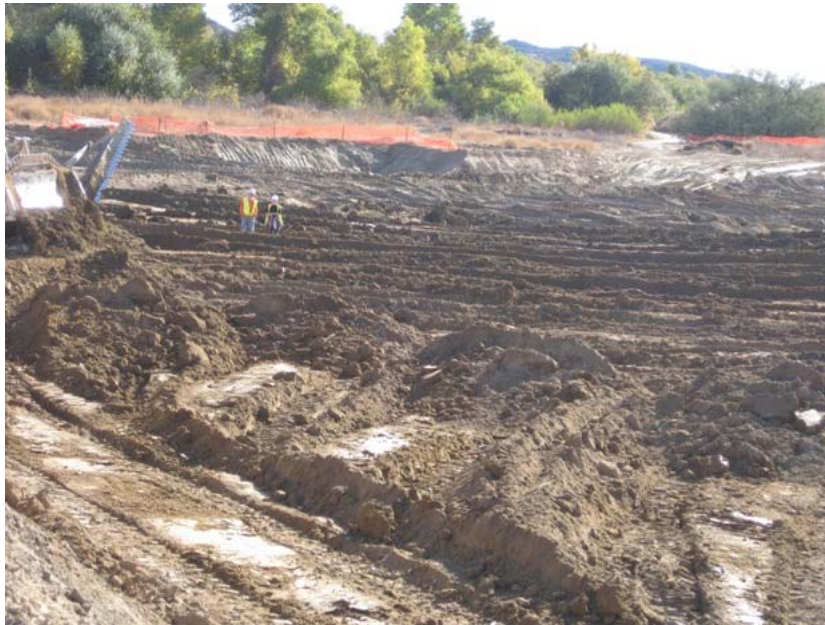
Figure 3: A second over-excitation area further eastward was being excavated during the subject week. The photograph faces northeastward.
