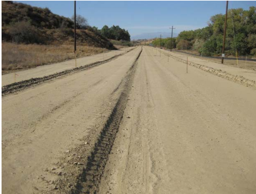
Figure 1: Rough grading of the new access road to the El Casco Substation has been completed. The notch in the center of the road will be filled with gravel. The photograph faces westward.
