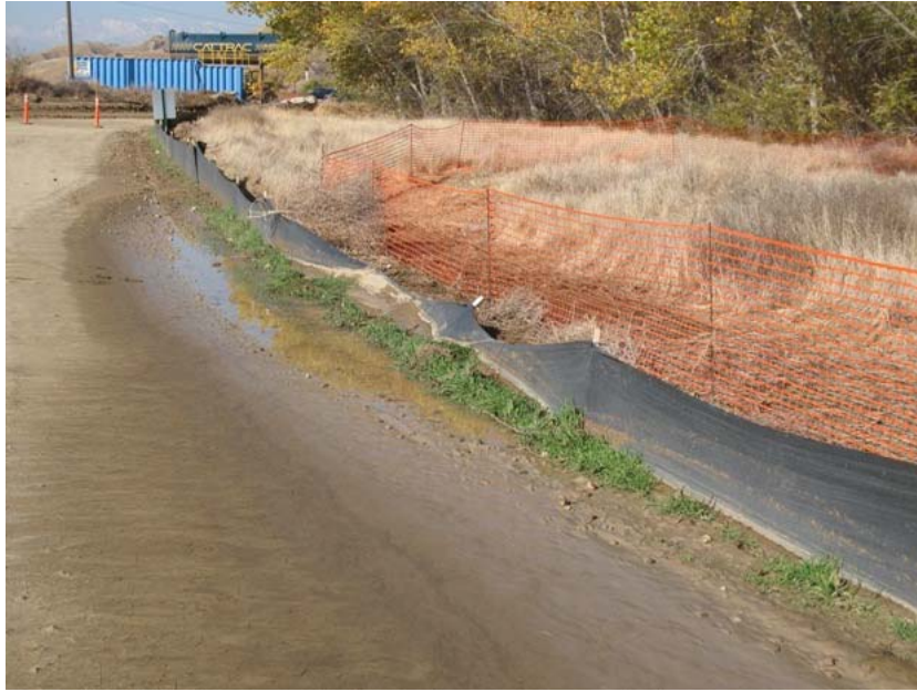
Figure 1: Several significant storm events occurred during the subject week. At El Casco Substation site the silt fencing along the pre-existing access road collapsed at one location. This section subsequently was repaired, and reinforced with sand bags. San Timoteo Creek, on the right, did not receive any siltation from the substation construction site. The orange fencing delineates a smooth tarplant population site. The photograph faces northwestward.
