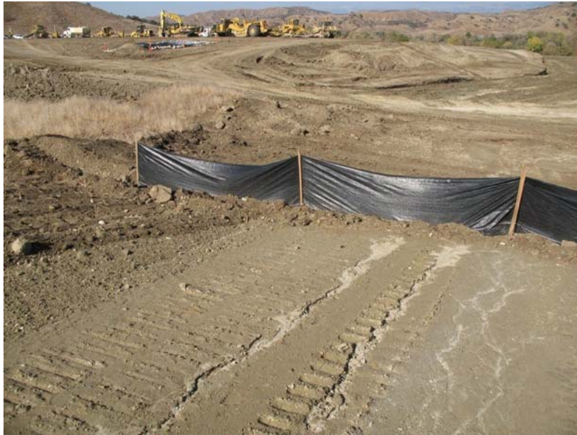
Figure 4: Additional silt fencing was placed where needed during the storm events of the subject week. No significant run off water or silt reached San Timoteo Creek from the substation construction site. The photograph faces northwestward.
