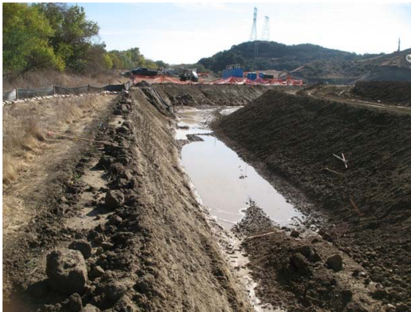
Figure 3: The over-excavation areas served to retain run off water. The silt fencing that had been moved closer to San Timoteo Creek to provide room for the over-excavation activity can be seen on the left. The photograph faces eastward.
