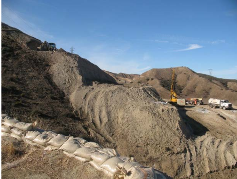
Figure 3: The upper five terrace systems on the higher western ridge have been completed. The contractor has temporarily skipped the sixth terrace location (middle empty bench) and worked on the seventh terrace (with the drill rig on the right) during the subject week. The photograph faces southward.
