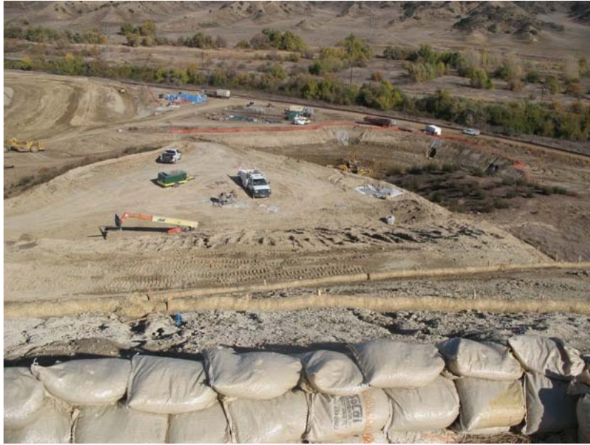
Figure 1: The westernmost over-excavated area (in the mid-distance to the left of the blue tank) has been over-excavated, lined with water resistant fabric and an underlying gravel blanket, and is being filled with firm material. A second over-excavation area further eastward (in front of the orange fencing) continued to be excavated during the subject week. The photograph was taken from one of the upper terraces and faces northward
