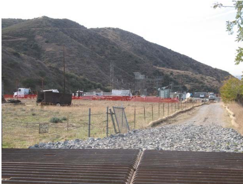
Figure 4: Construction at the Zanja Substation began during the prior week. Construction will consist of paving the access road, expansion of the substation perimeter fence (behind the orange fencing), placement of additional electrical equipment, and construction of a tower. Note the shaker plate, gravel bed, and erosion control straw wattles on the access road. The photograph faces westward.
