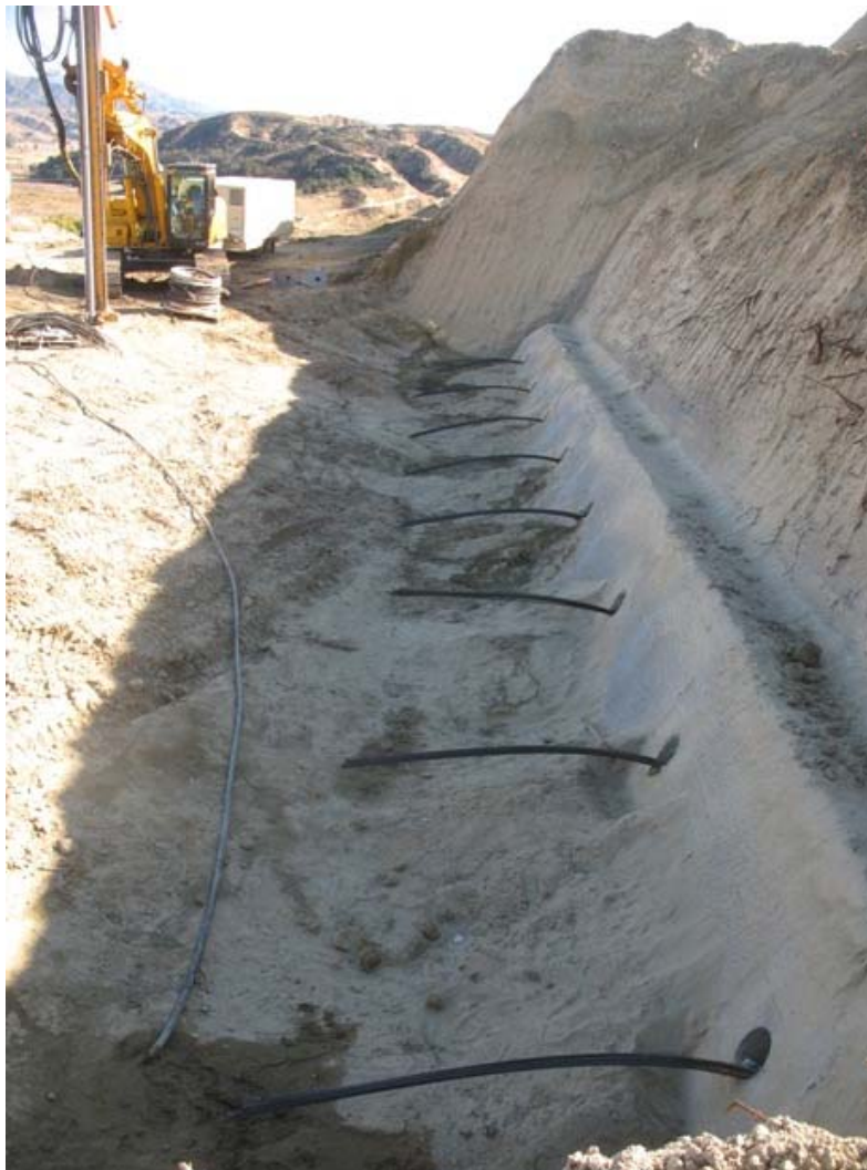
Figure 2: A tie-back wailer structure was under construction on the face of one of the terraces. The ends of the approximately 120-foot-long cable anchor can be seen emerging from the oblique bores dug into the hill. After completion of the wailer, the cables will be placed under tension.
