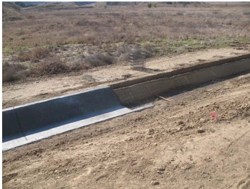
Figure 2: Concrete placement in the V-ditch alongside the El Casco Substation began during the subject period.
