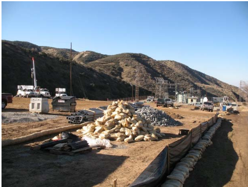
Figure 4: Construction continued during the subject period on the expansion and upgrading of the Zanja Substation (in the distance). The slope east of the substation has been removed in preparation for the expansion and has been spread on adjacent SCE land in the foreground where construction materials are being stored. The photograph faces westward.
