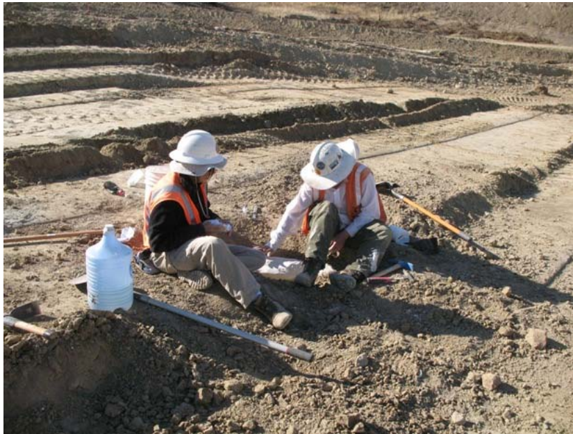
Figure 5: During the subject reporting period, fossils continued to be located, recovered, and processed at several locations at the El Casco Substation site. When fossils were discovered, construction activity was temporarily diverted to other areas, while paleontologists packaged and removed the fossils. Also material samples were collected from discovery sites. These samples were then processed by wet screening to uncover small and difficult to detect fossil material. In this photograph, a large mammal bone fragment has been packaged for removal.
