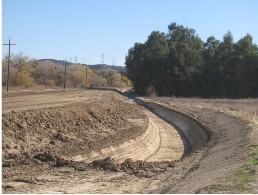
Figure 1: A V-ditch is being constructed on the south side (uphill) of the new El Casco Substation access road. The photo faces eastward.
