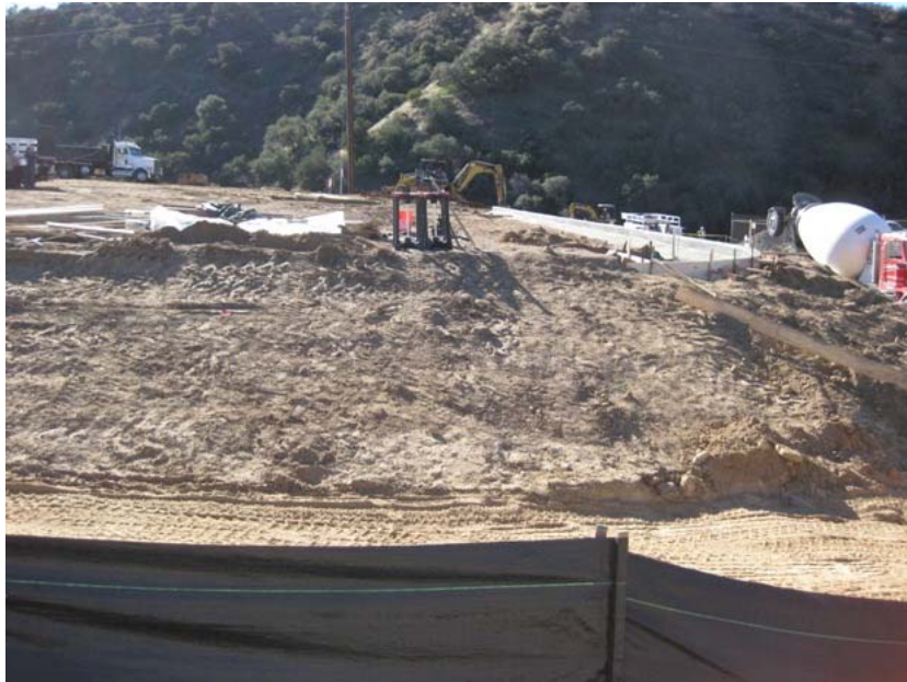
Figure 5: At Zanja Substation, the spoils from the berm excavation for the expansion of the station have been spread over an adjacent field, which appears to be used as a staging area. The photograph faces southward. The existing substation is to the right of the photograph.
