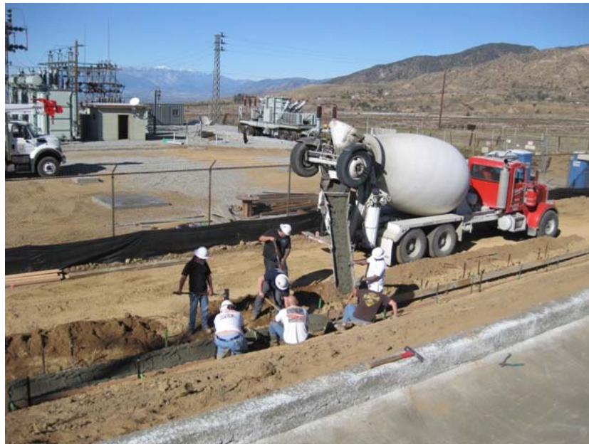
Figure 2: At Zanja Substation, drainage culverts were being built to the east of the proposed eastern expansion of the substation. The gravel blanket has been removed from the eastern portion of the substation (in middle distance) in preparation for construction. The photograph faces northwestward.
