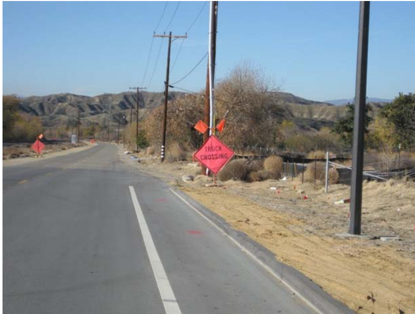
Figure 4: The entrance to the mobile water tower next to San Timoteo Canyon Road north of El Casco Substation (to the right of the photograph) is now marked with safety signs, as is San Timoteo Canyon Road for considerable distance in both directions from the entrance. The photograph faces westward.
