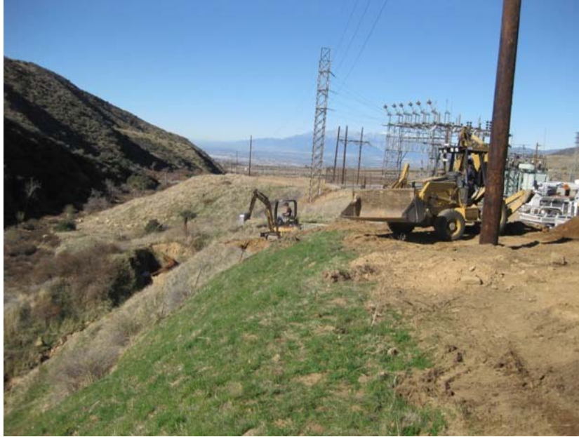
Figure 3: At Zanja Substation, erosion control measures were applied to the slope between the new power pole that was previously installed outside the existing station and the ravine to the south. The photograph faces westward.
