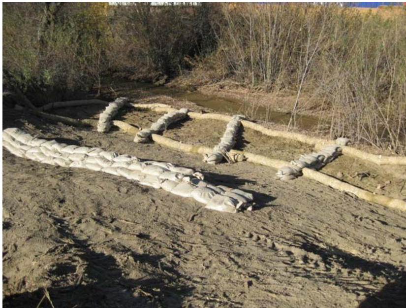
Figure 6: At El Casco Substation, riparian vegetation was cleared to the edge of San Timoteo Creek in preparation for the building of a concrete baffle which will direct and reduce the flow of run-off water (see Figure 1) to the creek. In anticipation of predicted winter storm events, the cleared riparian area was fitted with a network of straw wattling and sandbags during the subject week to prevent erosion in case the creek rises before the baffle structure can be built.
