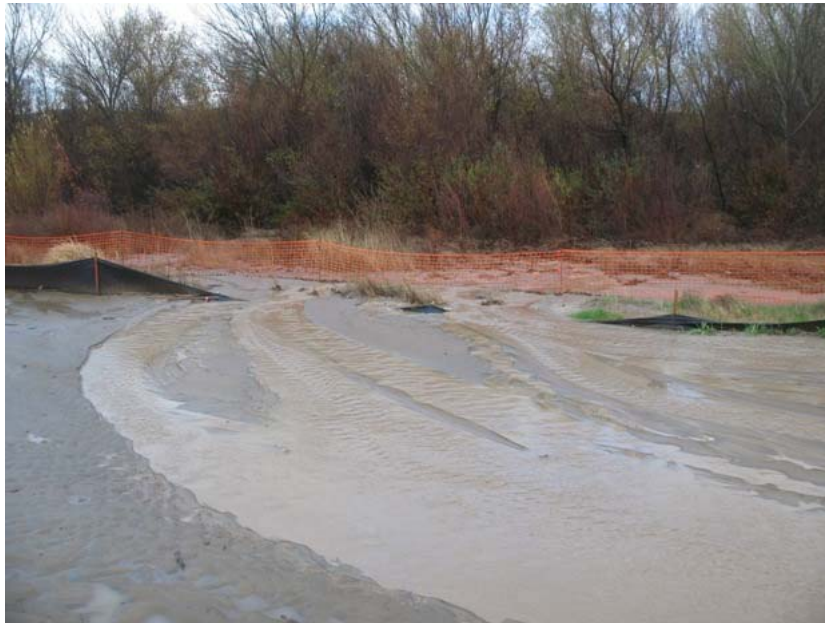
Figure 2: Silt fencing and other erosion control devices were compromised in several locations at the El Casco Substation site. The photograph faces northwestward, with San Timoteo Creek in the background.
