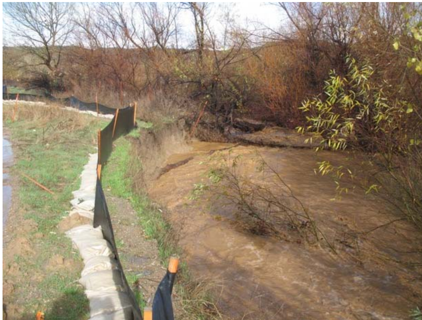
Figure 3: The swollen San Timoteo Creek eroded its bank, threatening to destroy some of the silt fencing at the El Casco Substation site. The photograph faces northwestward.
