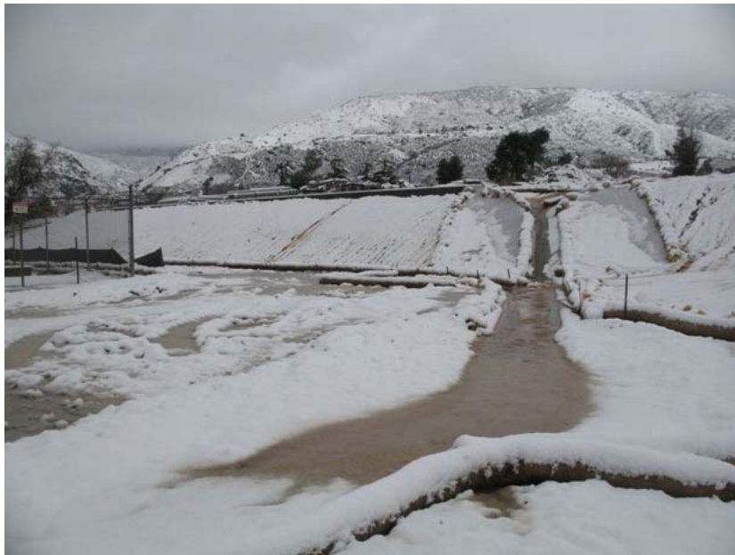
Figure 4: At Zanja Substation, erosion control measures were mostly effective, but some erosion gully formation was observed. In the photograph, which faces northeastward, runoff water is shunted around the substation (on the left) through two newly constructed V-ditches.
