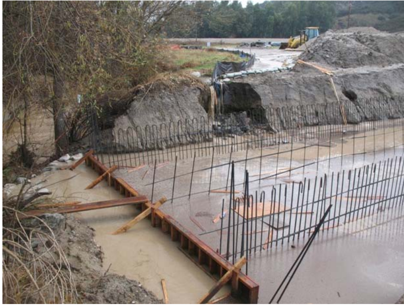
Figure 1: The partially completed box culvert at the El Casco Substation access road was inundated with stormwater, which then poured into San Timoteo Creek. The photograph faces southeastward.
