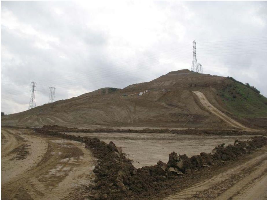
Figure 2: Work restarted on the western ridge terraces at El Casco Substation site. The photograph faces southeastward.
