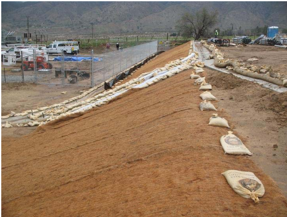
Figure 7: The newly installed V-ditches at Zanja Substation aided in controlling run-off during recent storms. The photograph faces northward.
