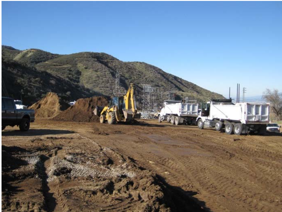
Figure 9: It has been determined that the disturbed area at the Zanja Substation work site has exceeded one acre and therefore requires a WDID permit from the State Water Resources Control Board. The photograph faces southwestward.
