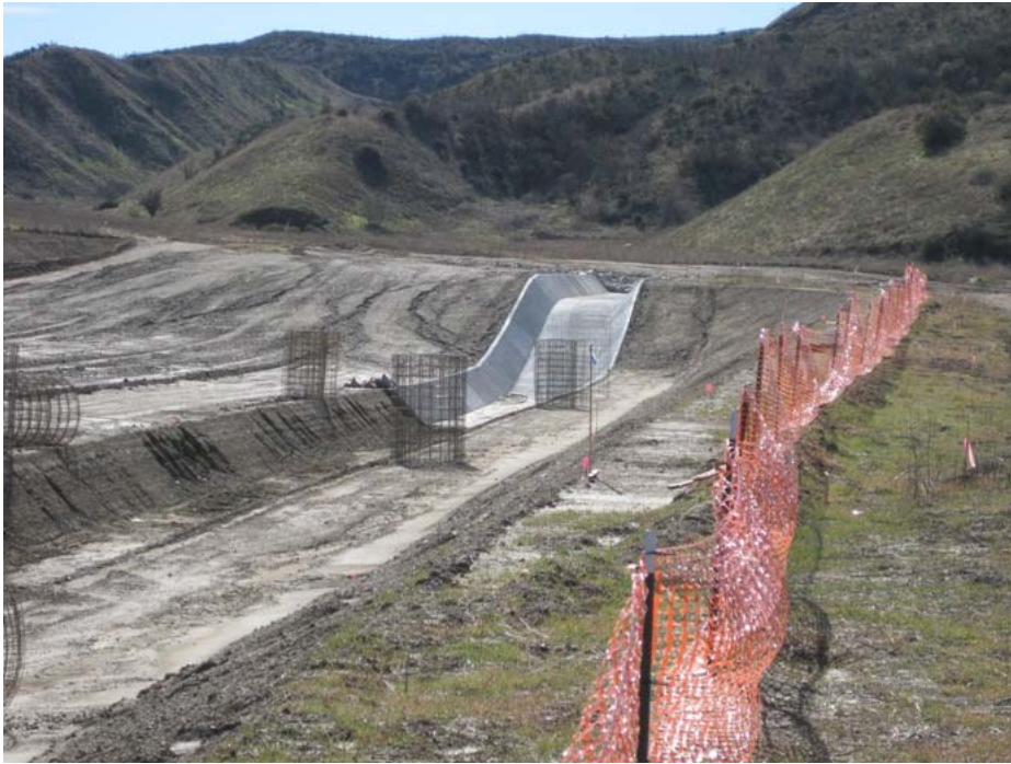
Figure 1: At El Casco Substation, work continued on the drainage ditch behind the office trailers. The photograph faces southward.
