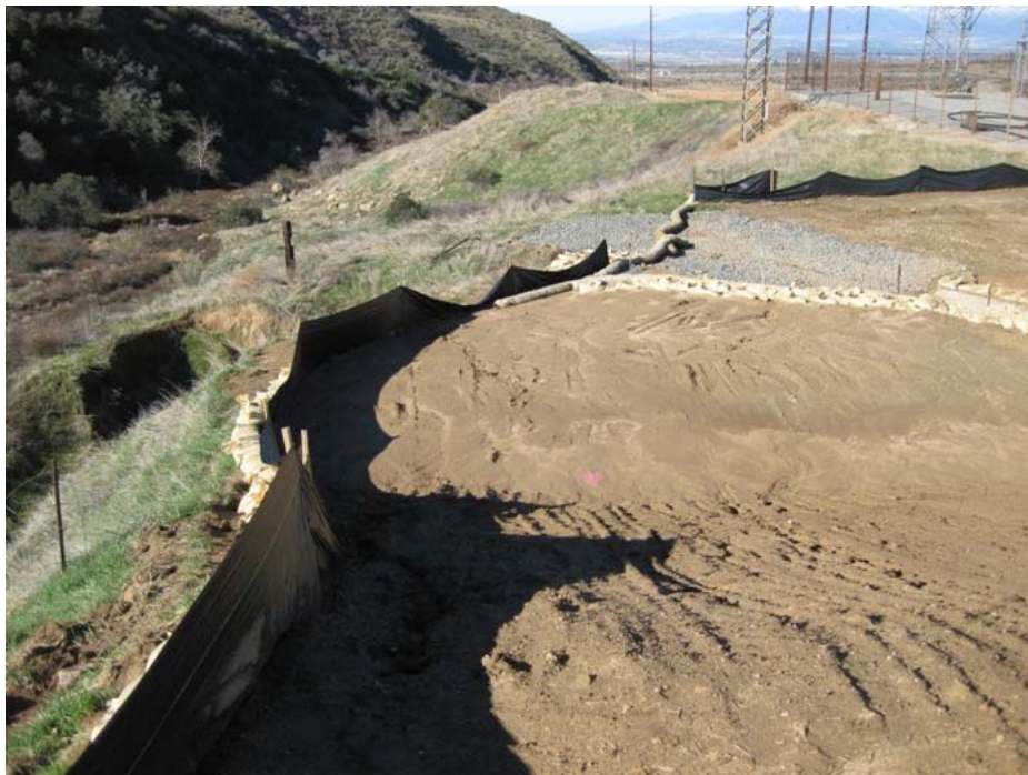
Figure 10: Erosion control devices prevented most siltation of a nearby watercourse during recent storms at Zanja Substation. The photograph faces westward.
