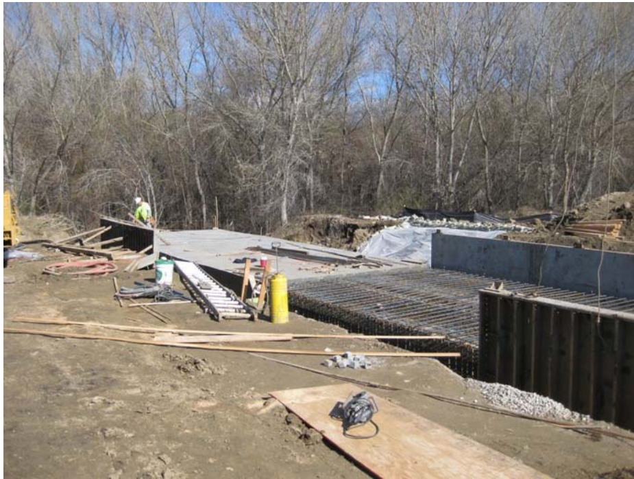
Figure 3: Concrete work restarted on the box culvert at the access road to El Casco Substation site. The photograph faces northward towards San Timoteo Creek.
