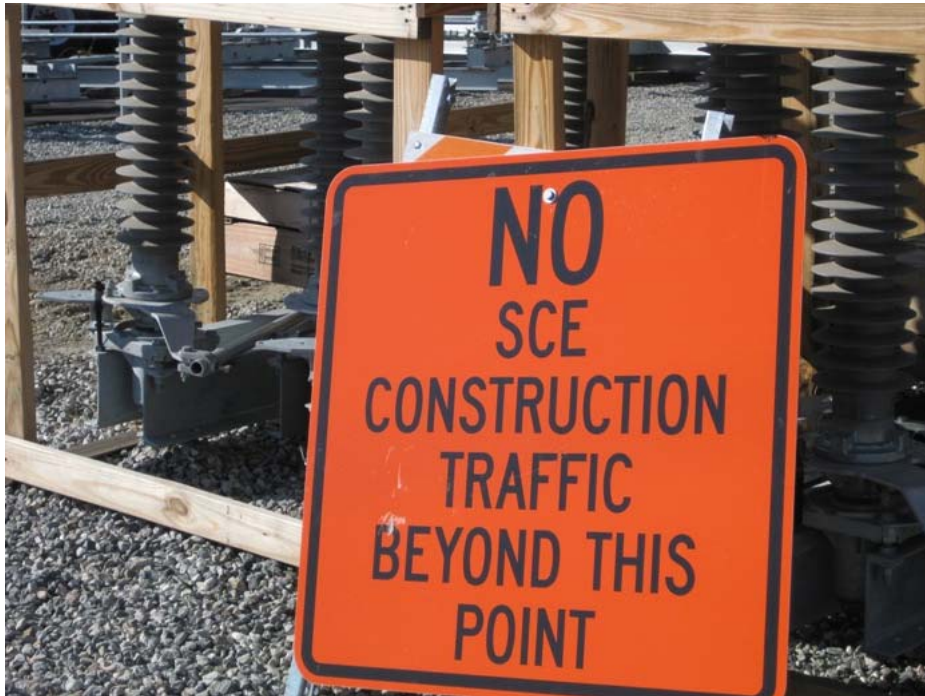
Figure 6: Signage was present on John street on the northern border of Banning Substation to restrict Project traffic to the commercial portion of the street.
