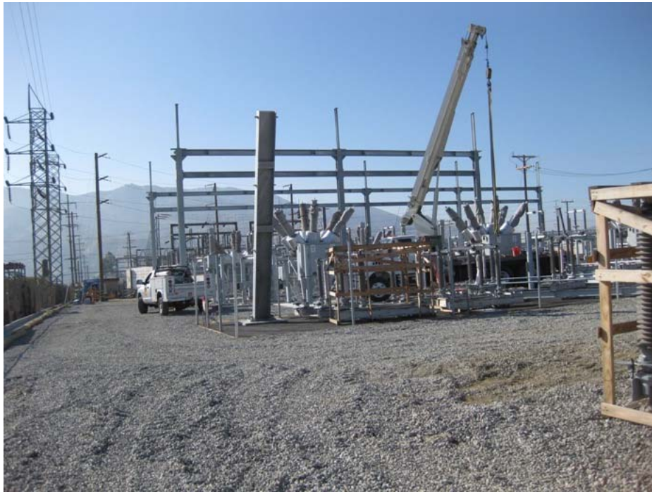
Figure 5: At Banning Substation, circuit breakers and other electrical equipment were installed in the northern portion of the substation site to house the expansion of the substation required by the El Casco Systems Project. The photograph faces southward.
