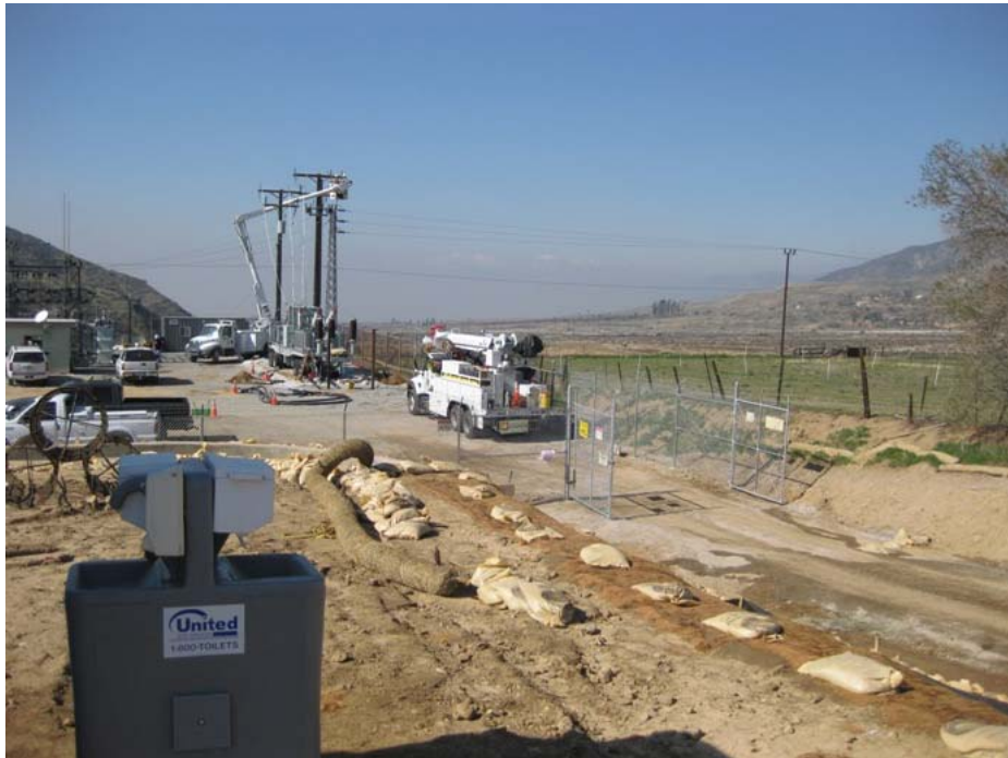
Figure 12: A TEWS request to allow distribution line crew access to set equipment on existing poles through an adjacent privately owned field on the northern side of Zanja Substation was requested by SCE and approved by CPUC. The photograph faces westward.
