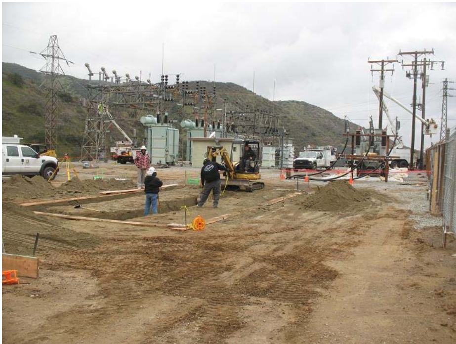
Figure 8: The foundation of the MEER building at the Zanja Substation being excavated. The photograph faces westward.
