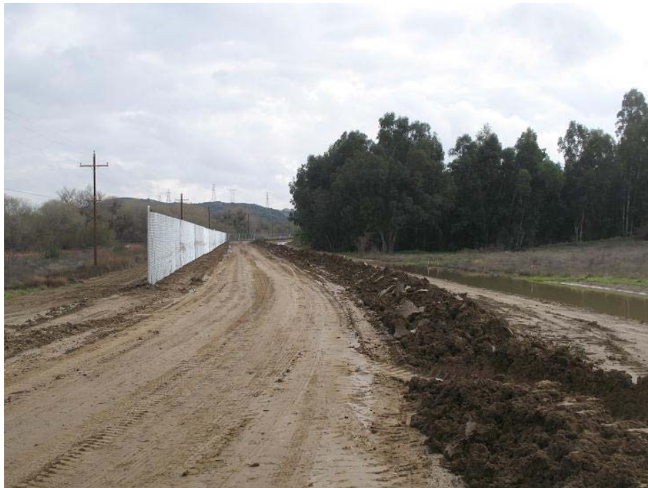
Figure 4: Chain link fencing was installed along the access road and substation pad. The photograph faces eastward towards the substation site.
