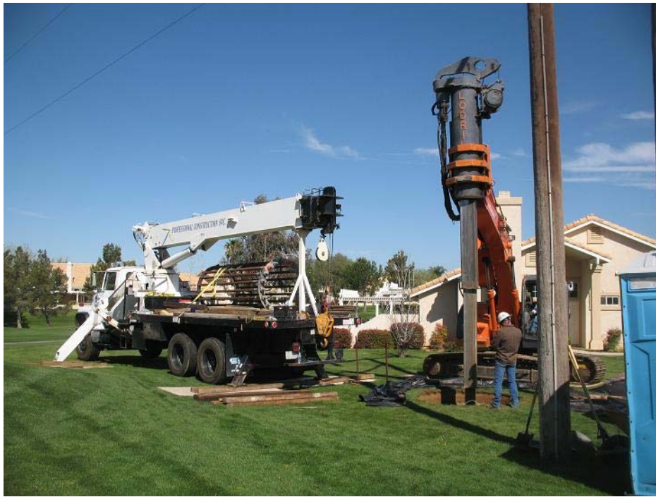
Figure 3: View of crews installing new pole foundations for Segment 3 of the sub-transmission line through the Sun Lakes development. The photograph faces northwestward.
