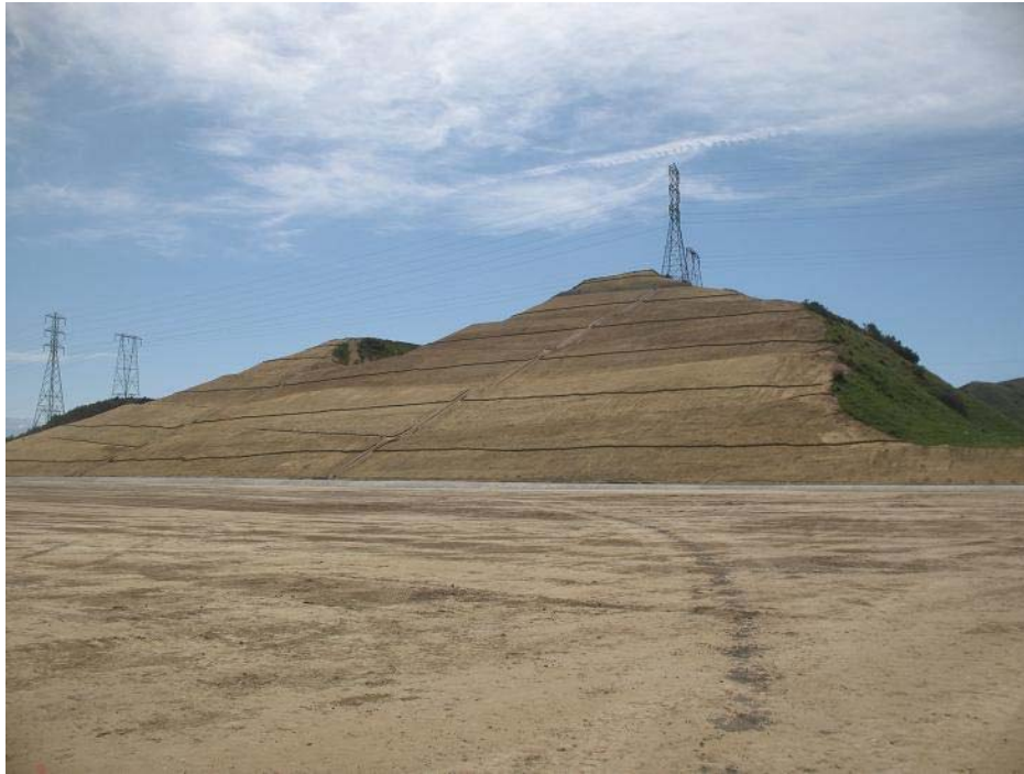
Figure 1: View of completed terraced slope at El Casco Substation. The photograph faces southeast.
