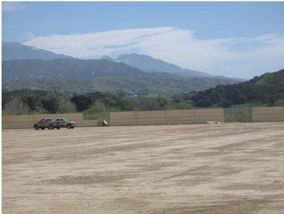
Figure 2: View of damaged sound barrier at El Casco Substation. The photograph faces northeastward.
