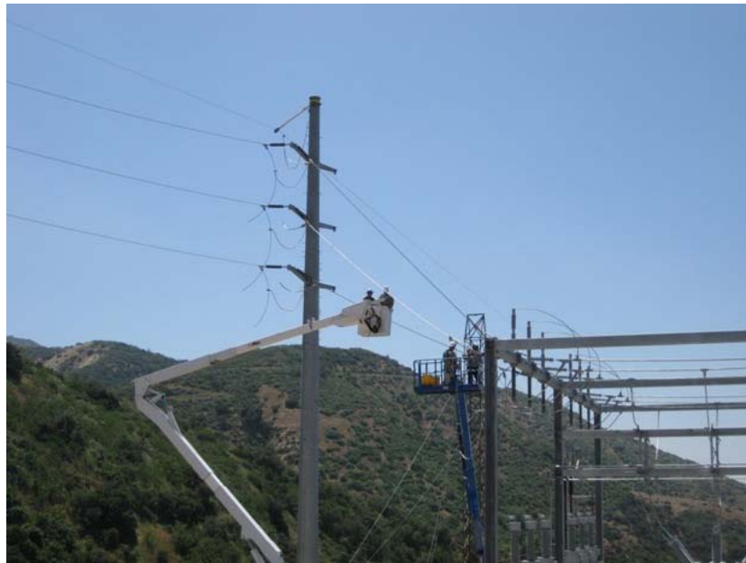
Figure 3: At Zanja Substation, most work on the upgrading of the substation has been completed. During the subject period electrical connections were made from adjacent poles to the substation in preparation for energizing of the substation in the near future. The photograph faces southwestward.
