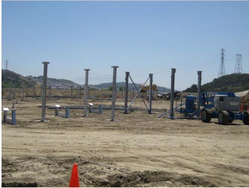
Figure 1: At El Casco Substation, construction of steel structures for the 220 kV portion of the substation began during the subject period. The photograph faces eastward.
