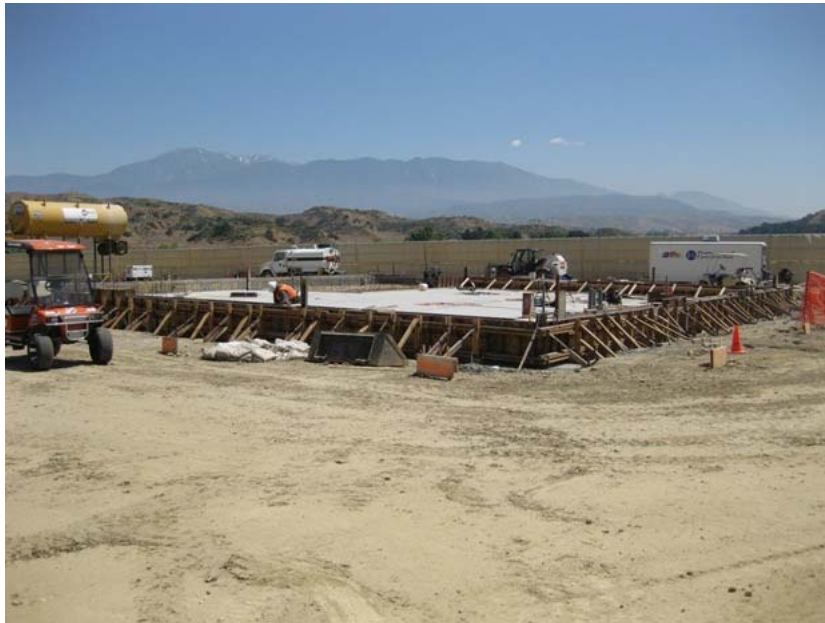
Figure 2: At El Casco Substation, building of the foundation for the 200 kV MEER began during the subject period. The photograph faces northeastward.
