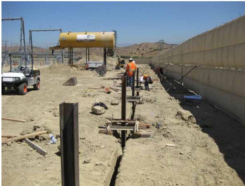
Figure 5: At the El Casco Substation site, construction began on the perimeter wall with the erection of support posts. After completion of the substation, the sound barrier to the right will be removed. The photograph faces northward.
