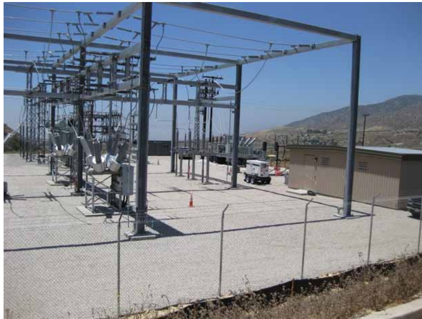
Figure 7: Construction activity at the Zanja Substation has been mostly completed. The new electrical system will be energized within a few weeks. After that event, the temporary mobile transformer (partially visible the MEER) will be removed. The photograph faces northwestward.
