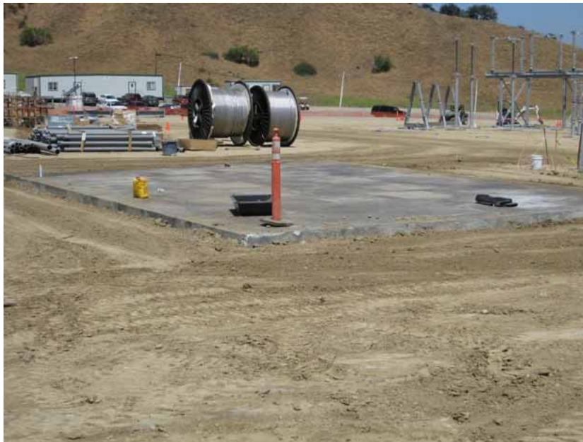
Figure 6: At the El Casco Substation site, one transformer pad was poured during the subject period. The photograph faces westward.
