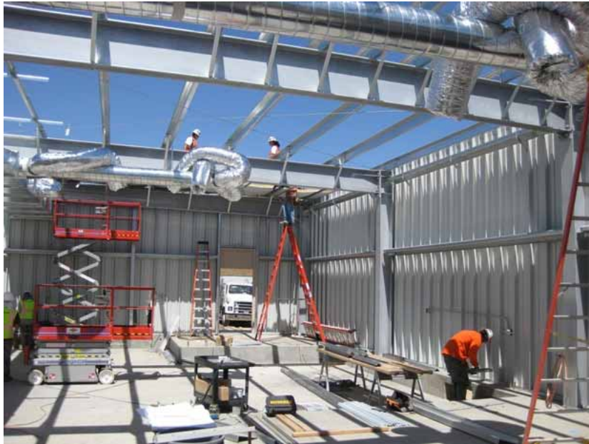
Figure 3: At the El Casco Substation site, construction of the 220/115 kV MEER continued.
