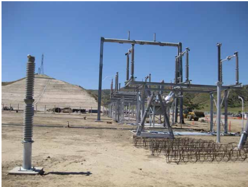
Figure 2: At the El Casco Substation site, work continued on the construction of steel structures for the 220 kV portion. The photograph faces southward.
