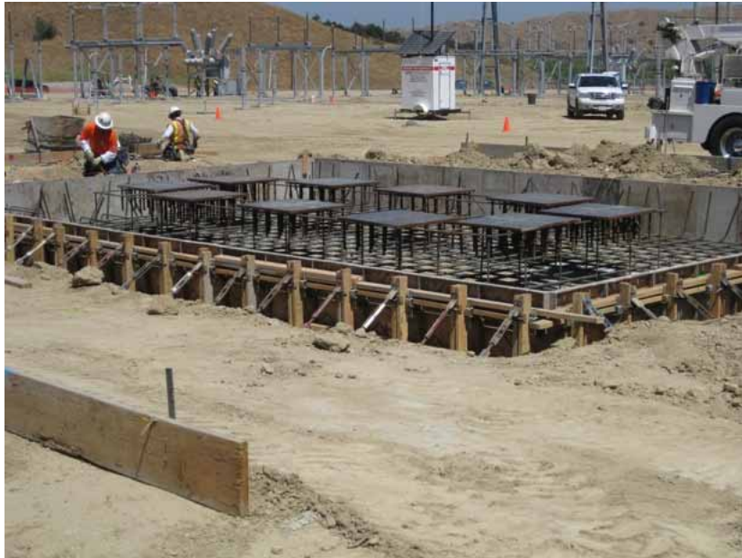
Figure 4: At the El Casco Substation site, construction of the 12 kV MEER continued. Seismic stabilizing devices were placed in the foundation. The photograph faces northwestward.
