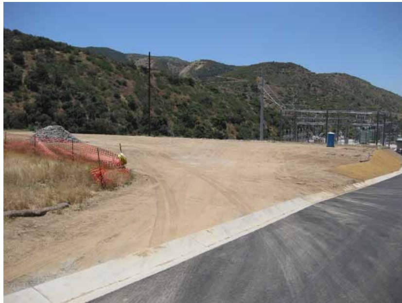
Figure 8: The staging area at Zanja Substation has been demobilized. It will be hydro-mulched for erosion control in a few weeks. Erosion control hydroseeding with a native plant mix will be applied to the staging area at the beginning of the next wet season. The photograph was taken from the newly paved access road, and faces southwestward.
