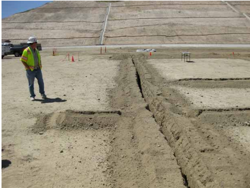
Figure 1: At the El Casco Substation site, the excavation of trenches for the grounding grid system continued. The photograph was taken in the 12 kV portion, and faces southward toward the stabilized hillside.
