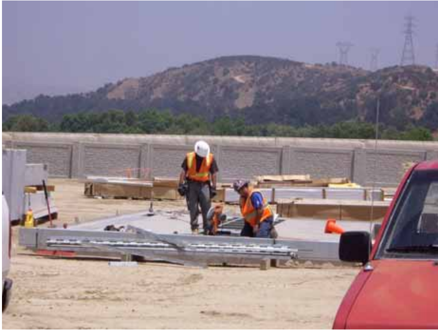
Figure 1: At the El Casco Substation site, crews worked on the concrete foundation for the 115 kV MEER building. This photograph is taken facing east.
