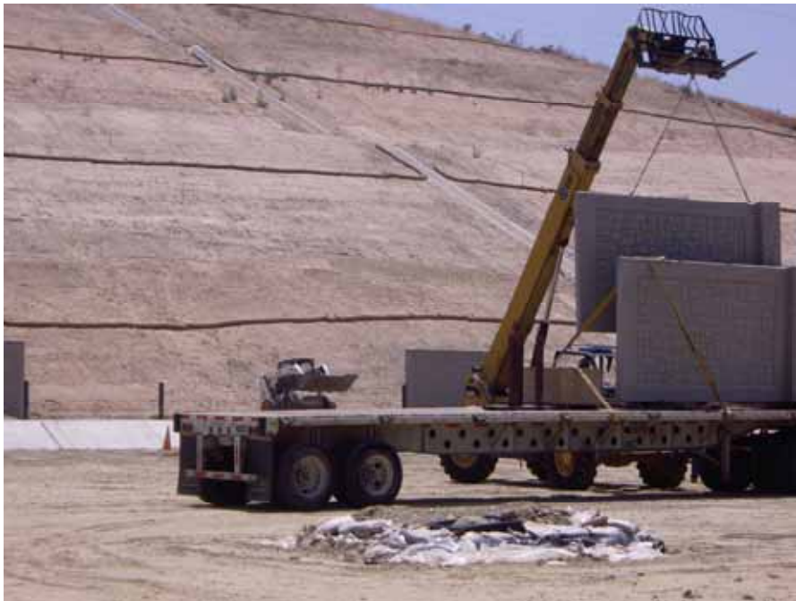
Figure 2: At the El Casco Substation site, a crane moved a perimeter wall panel. This photograph is taken facing south.
