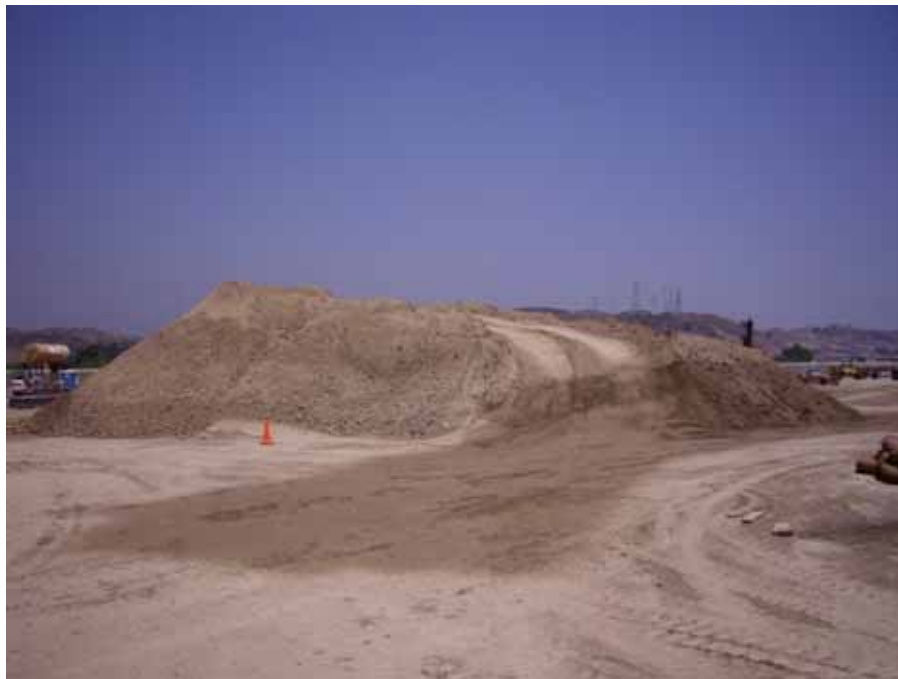
Figure 3: At the El Casco Substation site, a fill pile was generated from excavation for the perimeter wall. The photograph was taken when the pile had been recently watered.
