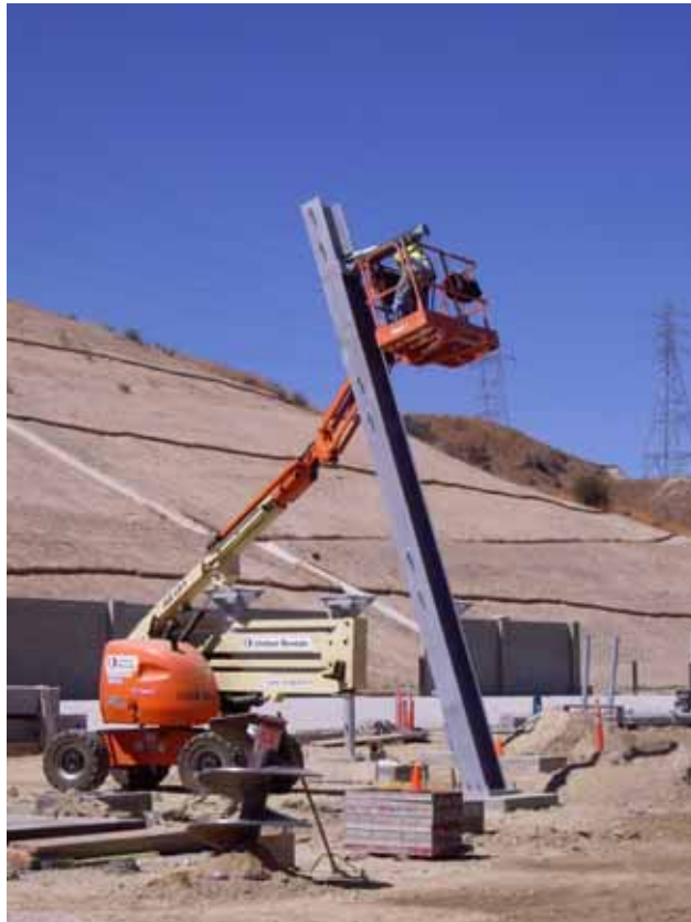
Figure 2: At the El Casco Substation site, crews worked on foundations for the AA banks for the 220 kV switchcracks. This photo is taken facing south.
