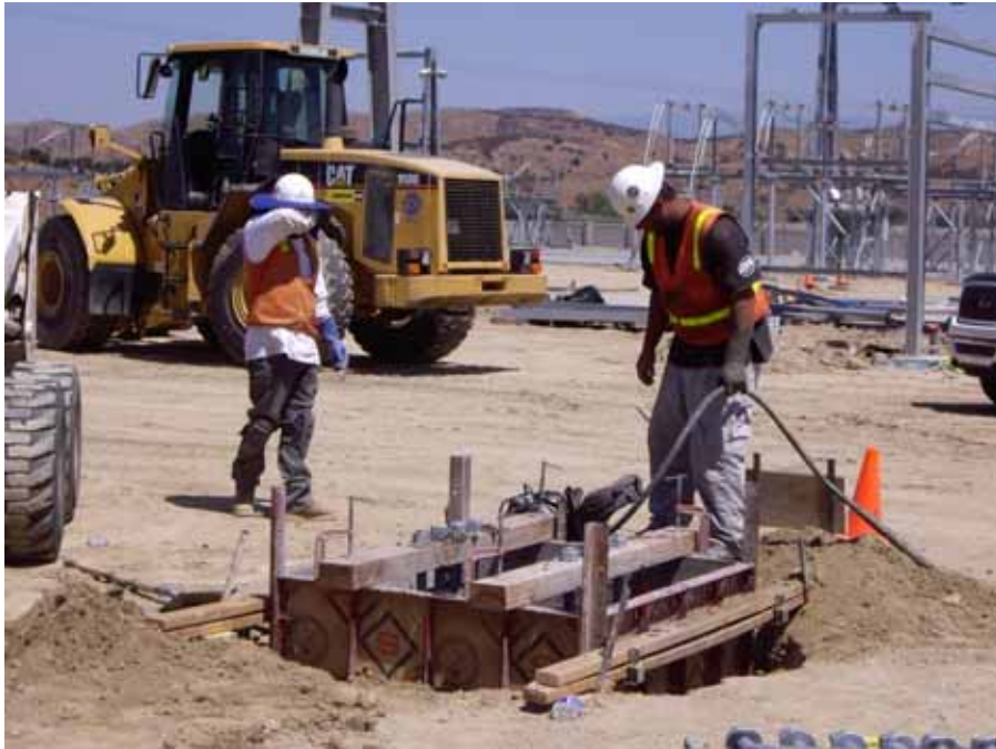
Figure 1: At the El Casco Substation site, crews worked on foundations for the AA banks for the 220 kV switchcracks.
