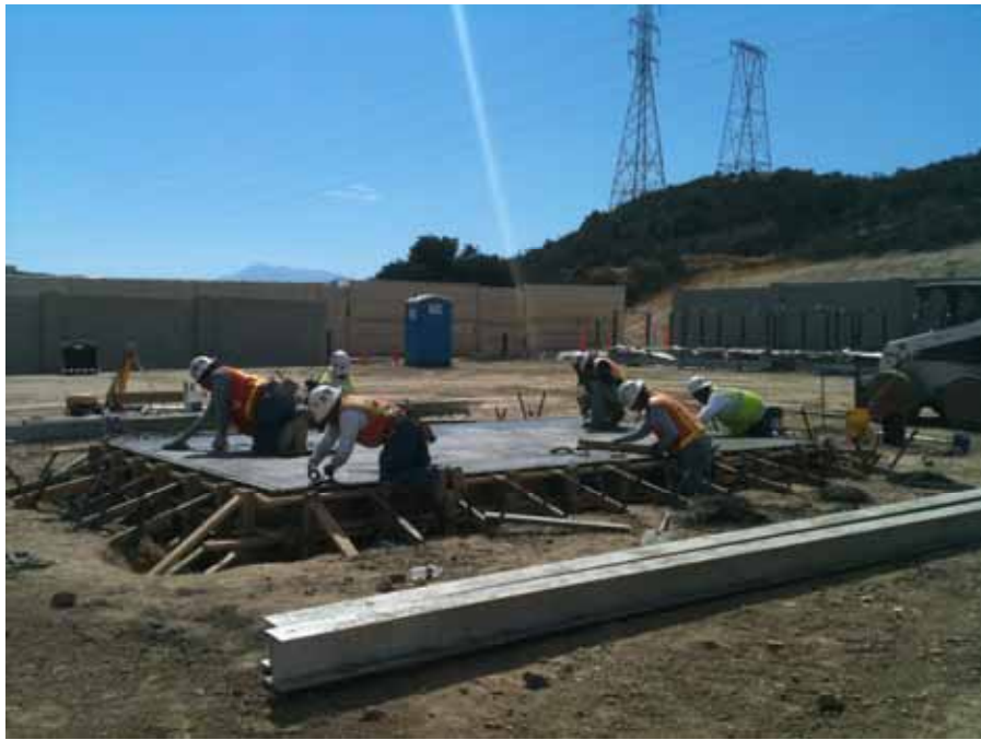
Figure 3: At the El Casco Substation site, work continued on the 115 kV MEER building. This photo is taken facing southeast.
