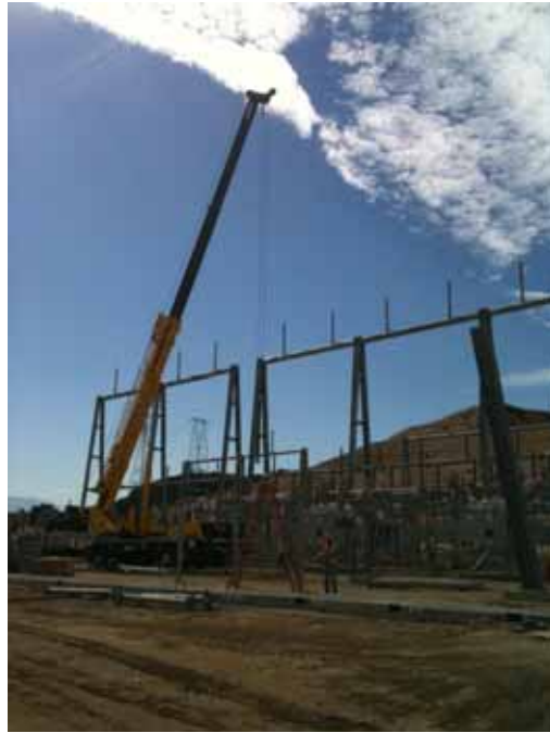
Figure 1: At the El Casco Substation site, crews worked on the AA banks for the 220 kV switchracks.
