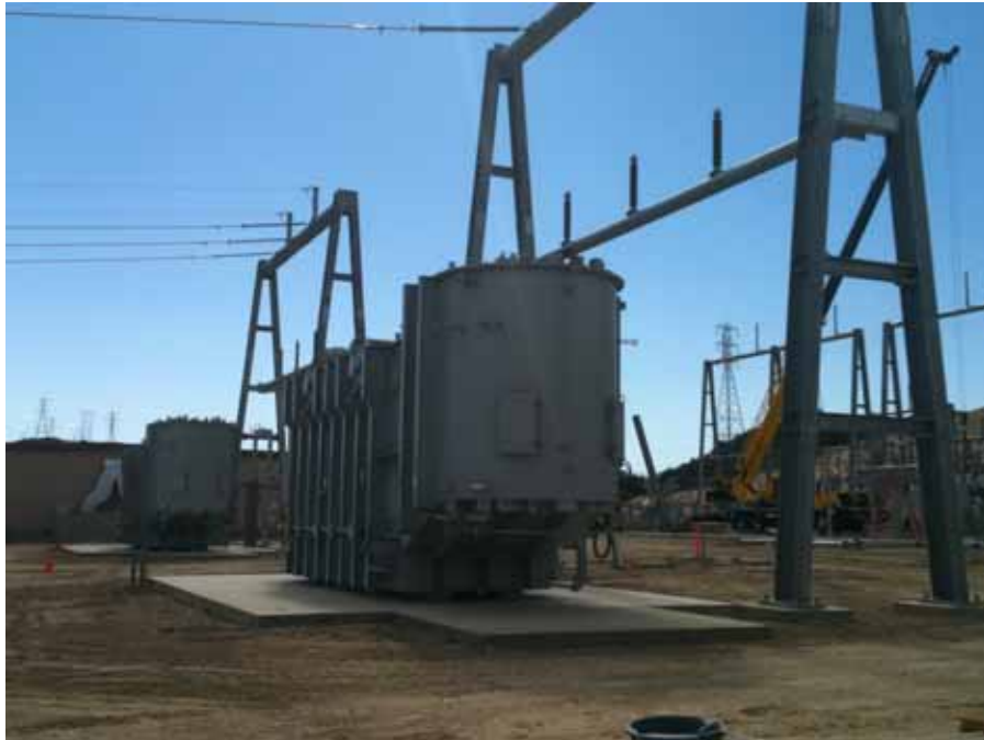
Figure 4: At the El Casco Substation site, a second 220 kV transformer was delivered on August 17 th .
