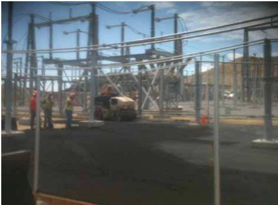
Figure 2: At the El Casco Substation site, paving occurred below the 220 kV switchracks.
