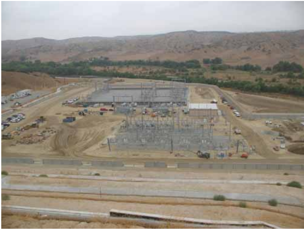
Figure 3: An overhead view of El Casco Substation taken from the southern slope that overlooks the project site.
