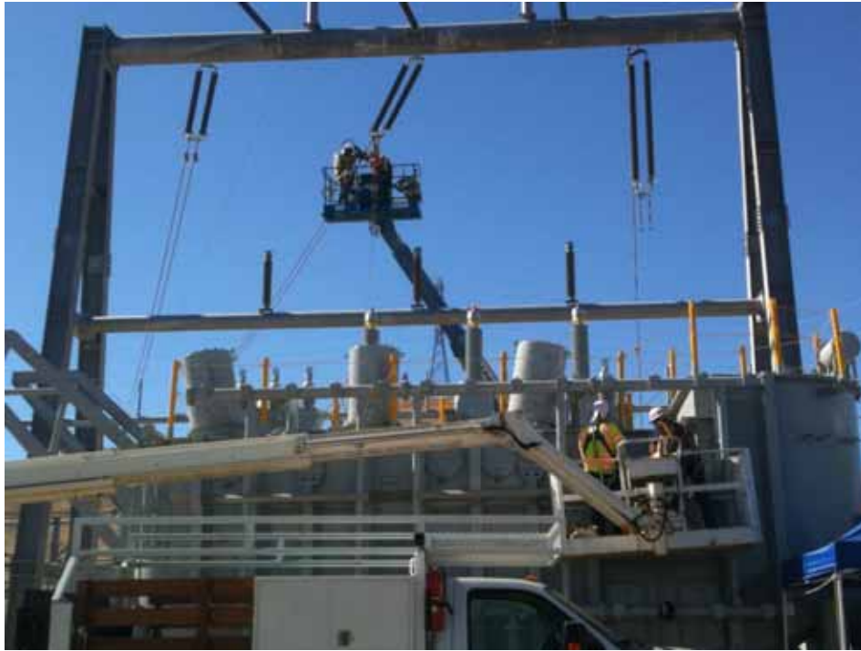
Figure 1: At the El Casco Substation site, crews worked on the AA banks for the 220 kV switchracks (background) and on one of the two 220/115 kV transformers (foreground).
