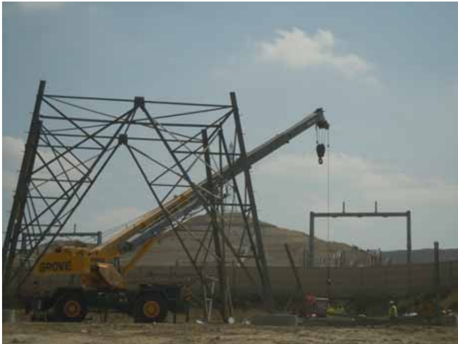
Figure 2: At the El Casco Substation site, crews work on assembling a distribution line tower.
