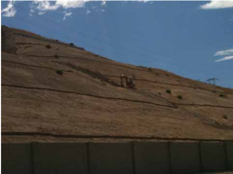
Figure 1: At the El Casco Substation site, crews worked on a trench for fiber optic cable on the southern slope of the site.
