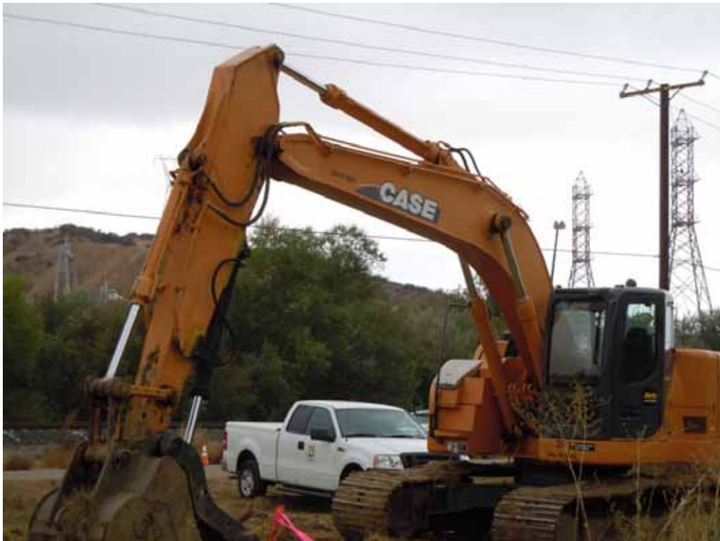
Figure 3: Outside the El Casco Substation site along San Timoteo Canyon Road, the excavator that was stolen/returned. The new ECS 220 kV towers are visible in the background. Picture is taken facing south.
