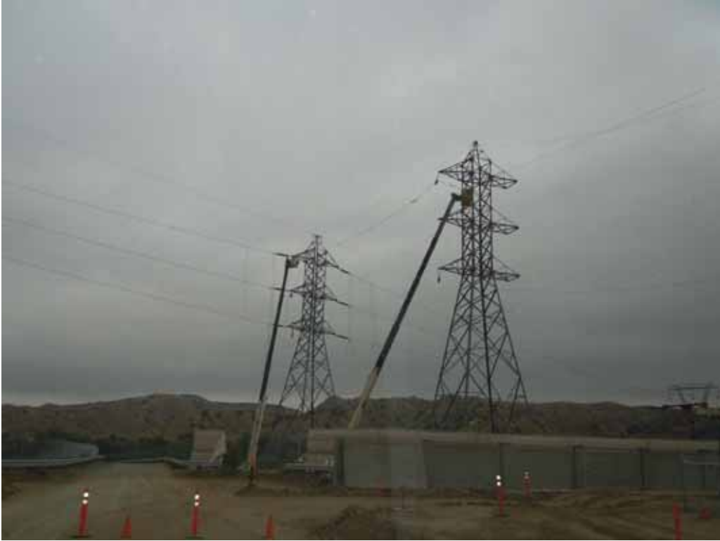
Figure 1: At the El Casco Substation site, crews worked on the 220 kV towers on the lower pad. Picture is taken facing north.
