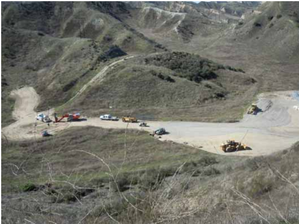
Figure 2: Crews worked on drilling a foundation for a TSP for the 115 kV subtransmission line, Segment 8.
