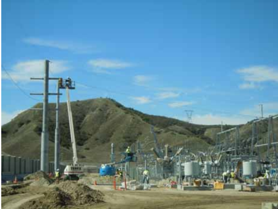
Figure 1: At the El Casco Substation site, workers strung wire on a TSP. The picture is taken facing west.
