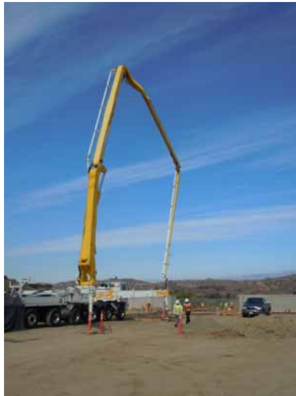
Figure 2: At the El Casco Substation site, workers pour concrete for the permanent access road.
