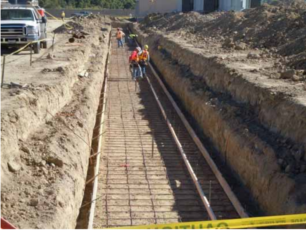
Figure 1: At the El Casco Substation site, workers work in a trench on the substation pad.
